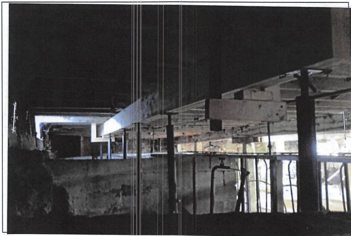
Photo # 16 Description: Failing North Sill – Temporary Stabilized (After) Photo 16 Temporary Stabilizer:
