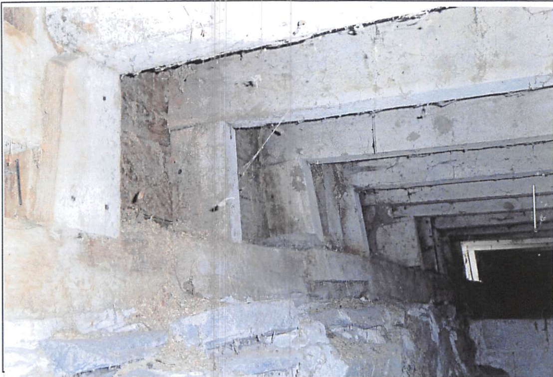
Photo # 15 Failing North Wall Sill (Before) Photo 15 Failing Sill North:
