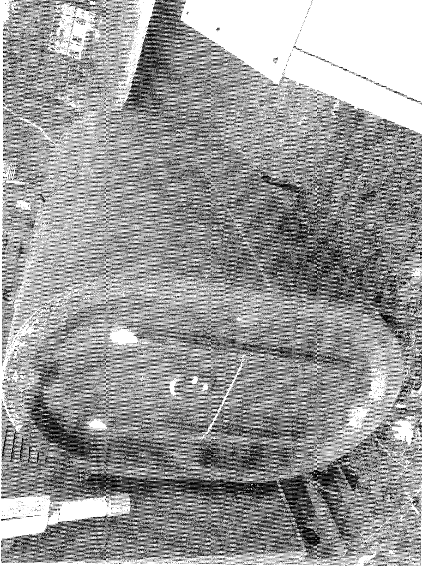
Two 275 gal fuel tanks,
