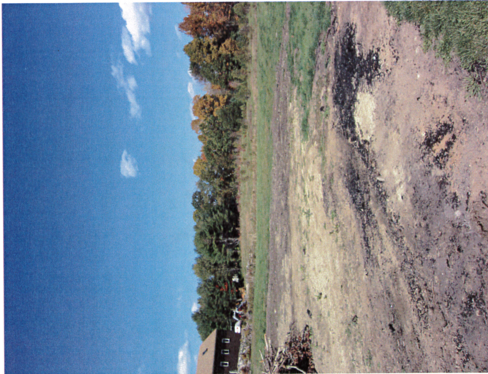
Photo 26: photo_Callahan_2014-10-09_26 Location Method: GPS Latitude: 43.00596 Longitude: -70.943581 Orientation: 356° Photograph Date: 10/09/2014 Photographer: Deborah Goard Description: From the approximate southeast corner of the Exclusion Area looking north northwest along the approximate boundary line. Note the areas used to burn brush is mostly within the Exclusion Area..
