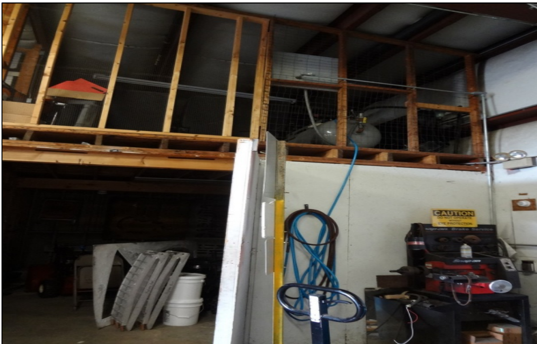
Storage Mezzanine. Note lack of proper handrail.
