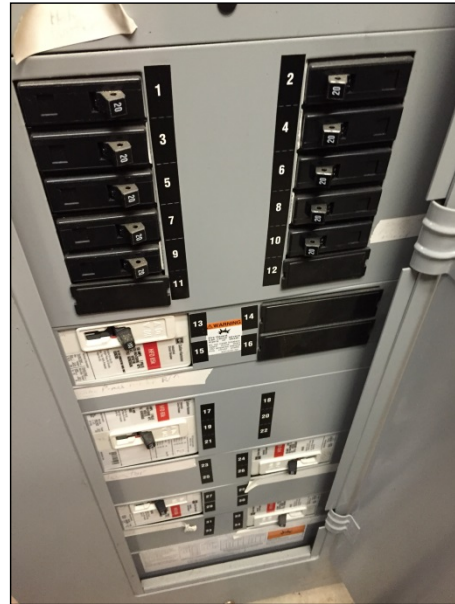
Main Electrical Service Panelboard
