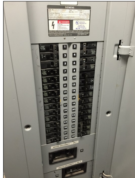
Main Electrical Service Panelboard
