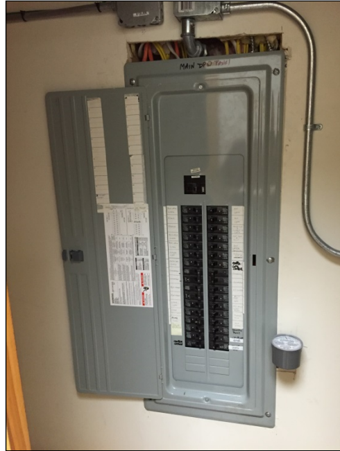
Main Electrical Service Panelboard
