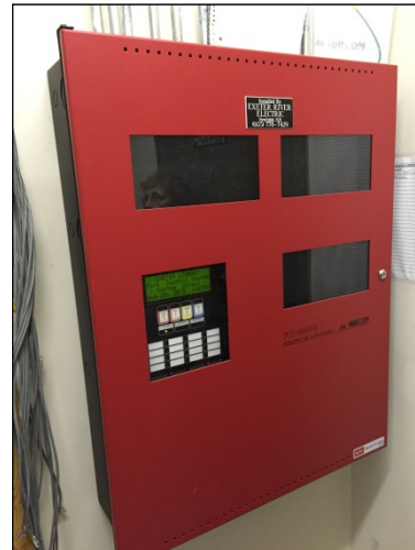
Existing Fire Alarm Control Panel
