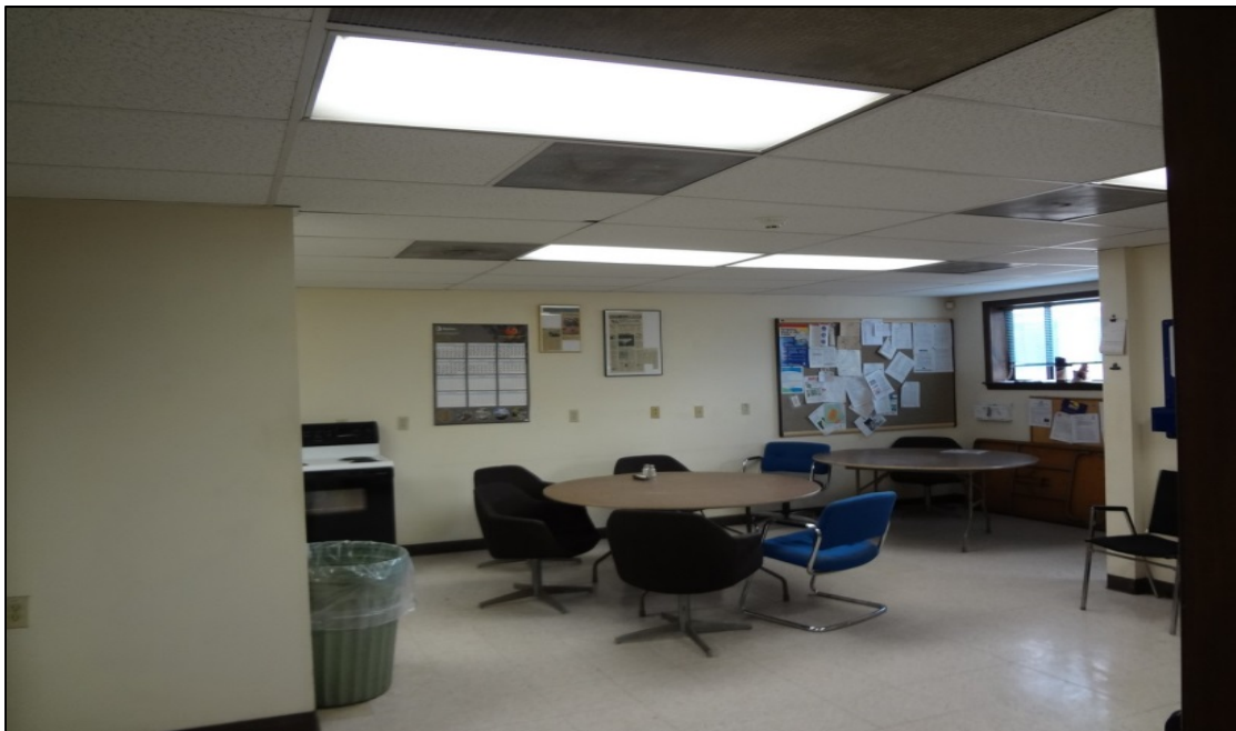
Break room. Note stove with no vent hood.
