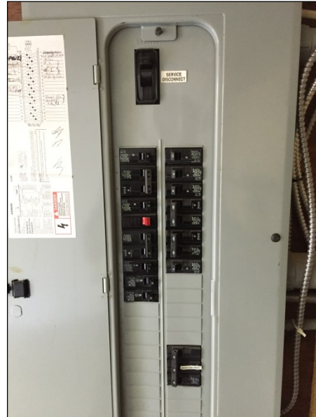
Main Electrical Service Panelboard
