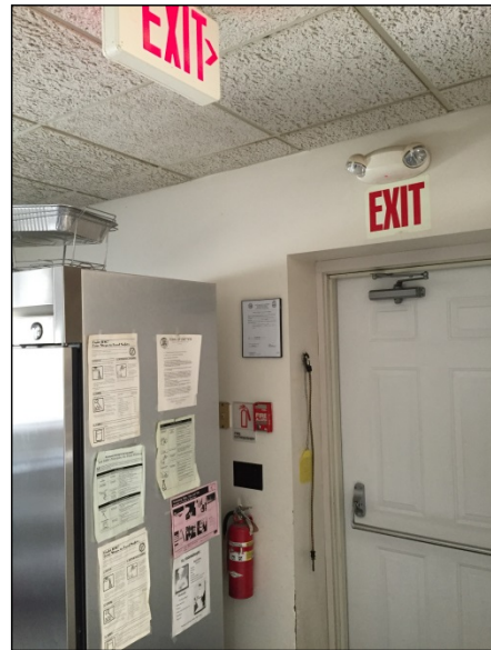
Exit Sign and Remote Battery Unit Heads
