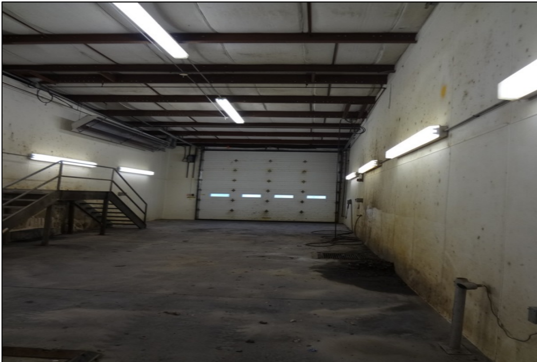
Wash-bay on east side of Water Department Garage. Note Infrared heating units on the wall.
