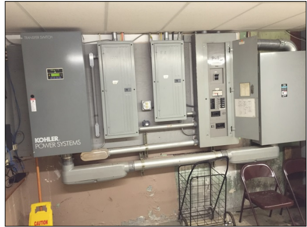
Main Electrical Service Lineup
