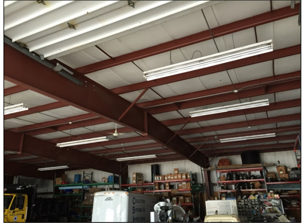
Pendant Mounted Fluorescent Fixtures
