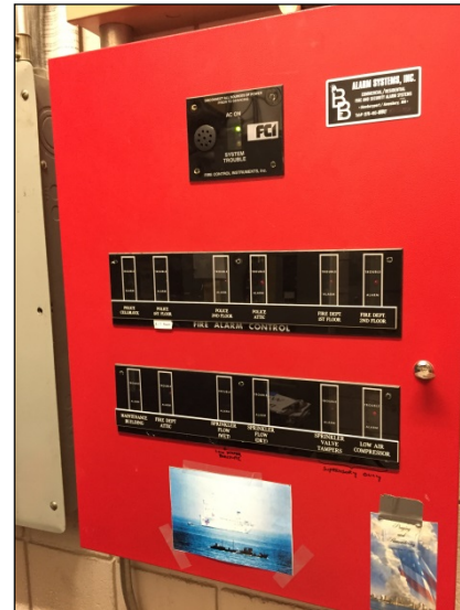
Existing Fire Alarm Control Panel
