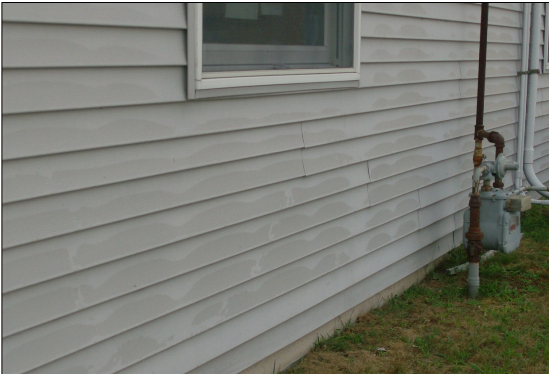
Condensation formed early morning on south side of building.
