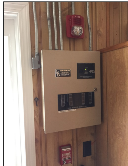
Existing Fire Alarm Control Panel
