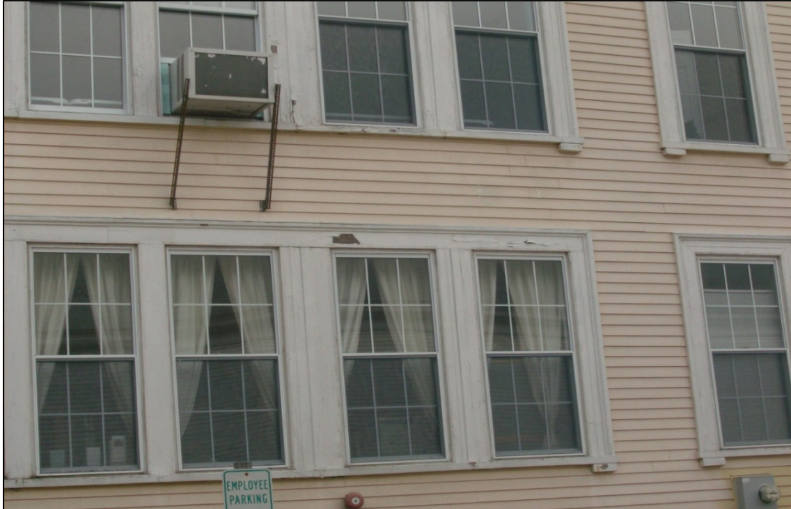
Peeling paint on trim, typical on all sides of the building (including some of the siding).
