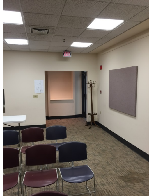
General Recessed Mounted Outlets
