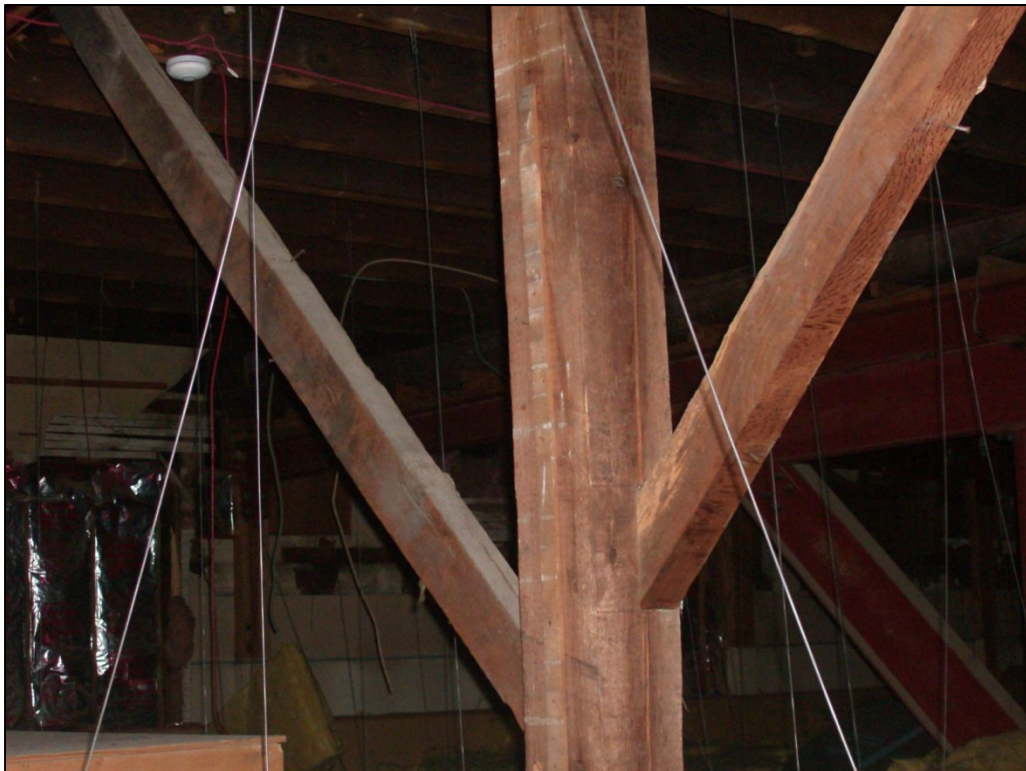
New framing in attic area above Senior Center. Note steel truss in background that was added when second floor walls and floor were removed, and the roof was lowered.
