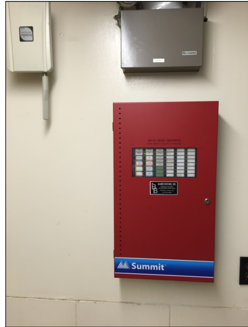
Existing Fire Alarm Control Panel
