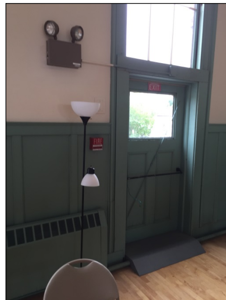
Existing Fire Alarm Pull Station
