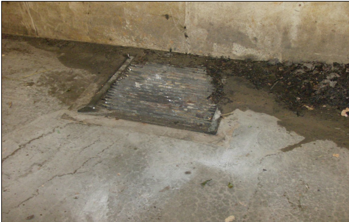
Wash-bay catch basin and accumulation of debris.
