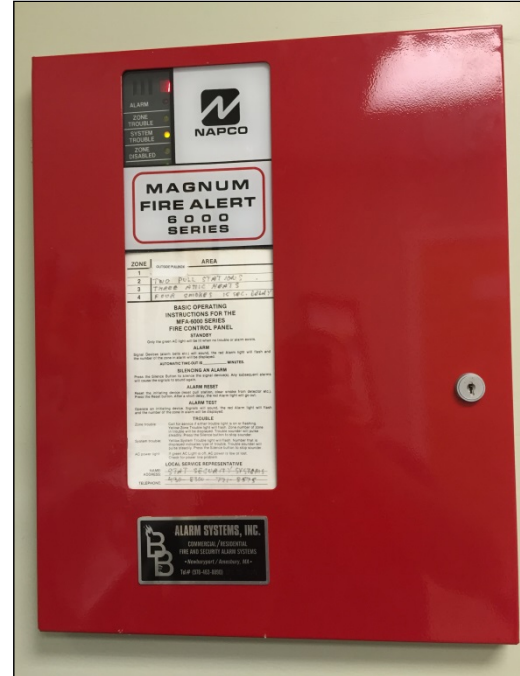
Fire Alarm Control Panel
