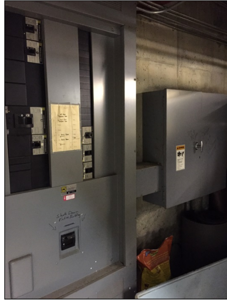
Main Electrical Service Panelboard
