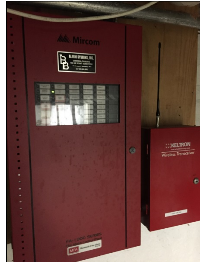
Existing Fire Alarm Control Panel
