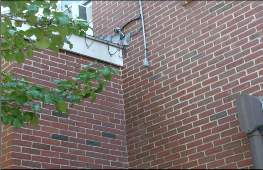
Valley over main entrance. Ice dams are a constant problem, note heat tape.
