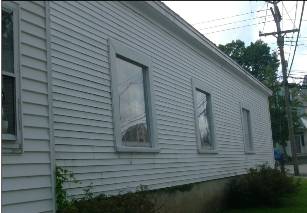
North wall of Fire Museum. Note plexi-glass panels over the original windows.
