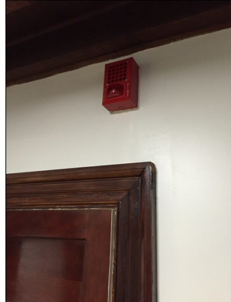
Existing Fire Alarm Audio Visual Device
