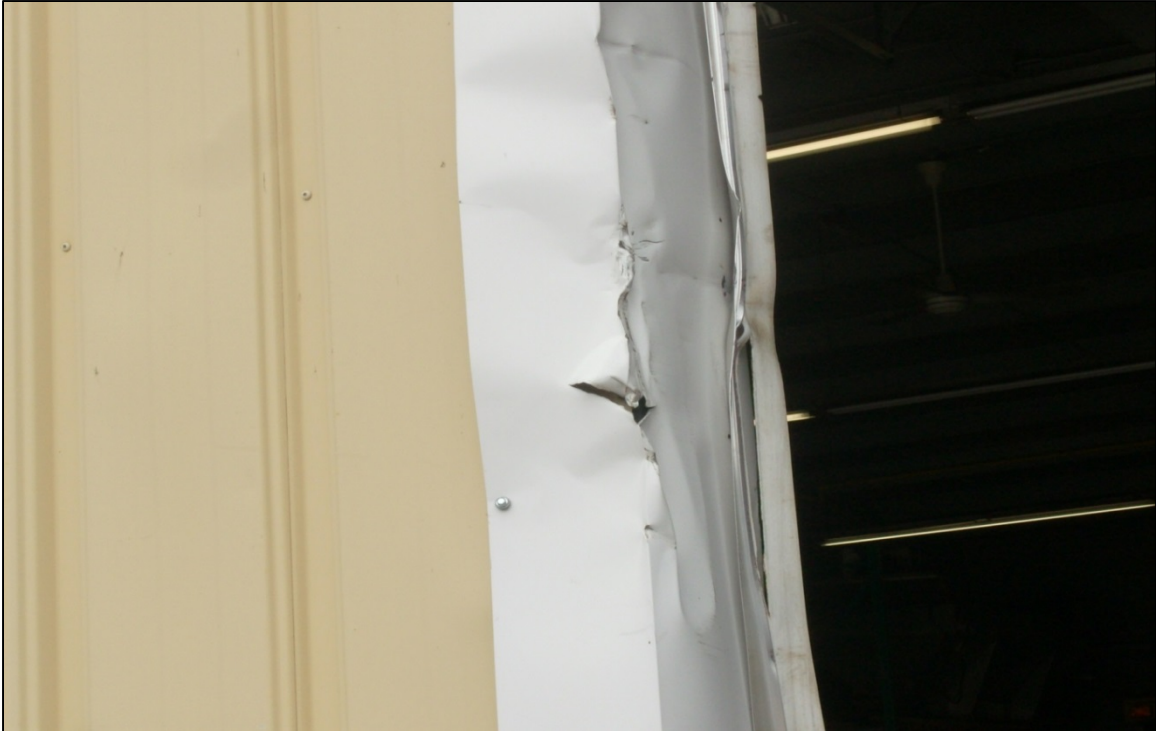
Damage to door jamb at one of the truck bays.
