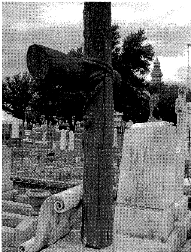
Figure 10. The sandstone cross (carved to look like wood) in this grave marker in St. Michael's Cemetery in Pensacola, FL, provides an example of inherent vice – the severe delamination affecting the sandstone has occurred along its natural bedding planes. Photo: Fran Gale.
