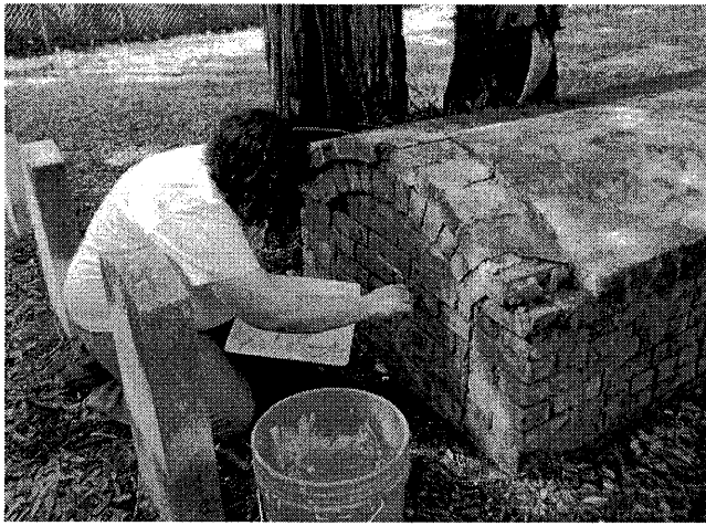
Figure 19. Masonry markers like this box tomb may require the repointing of mortar joints. It is important to use a mortar that is softer than the historic brick. In this case a conservator uses a lime putty-based mortar to repoint. Photo: Jason Church.
