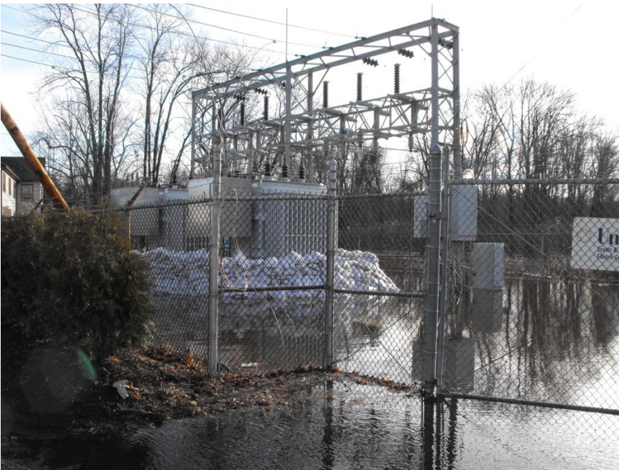
3-16-2010: Utilil Sub-Station on the Exeter River
