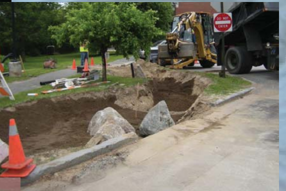
The Exeter Department of Public Works prepares the rain garden under the design and direction of Ironwood design group. Boulders slow water as it enters the garden off the steep hill of Chestnut Street. A special compost mix quickly infiltrates the the stormwater back into the groundwater table.
