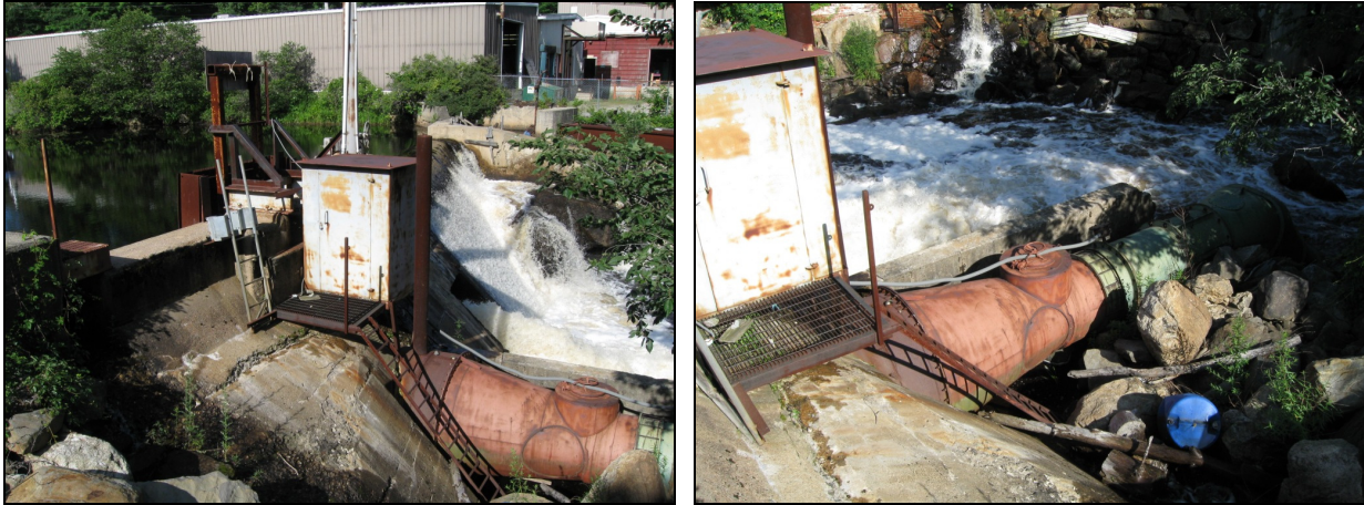
Brentwood Hydroelectric Dam and Turbine (2009)
