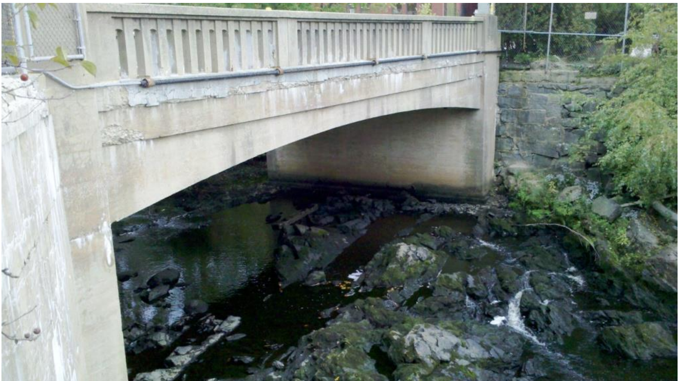
View of ledge outcrops under east of String Bridge (downstream of the dam), facing W
