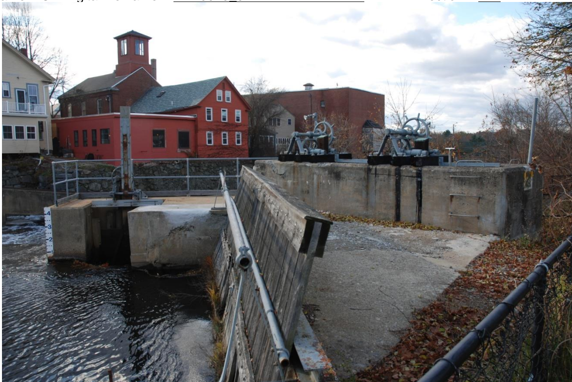
Photo # 5 Description: Low-level gate (center) and penstock baffle wall Roll and Frame # OR Digital file name: EXE0043_05 Direction: NW
