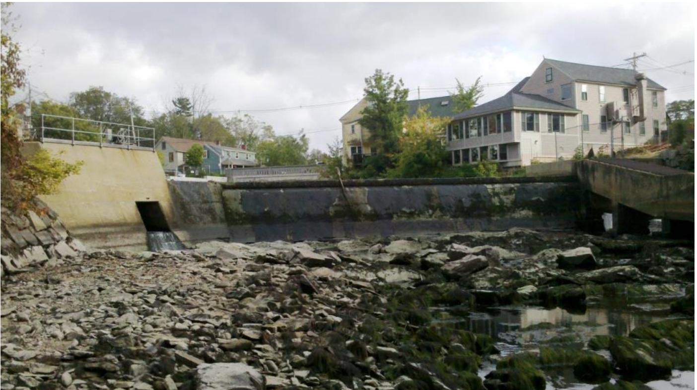
View of low-level gate (left), dam (center), and fish passage (right), facing S
