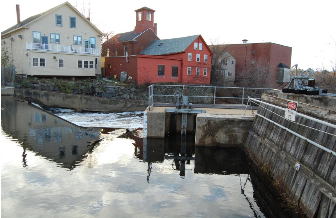
Photo # 3 Description: Fish passage (left) and penstock baffle wall (right) and low-level gate (center) Roll and Frame # OR Digital file name: EXE0043_03 Direction: NW
