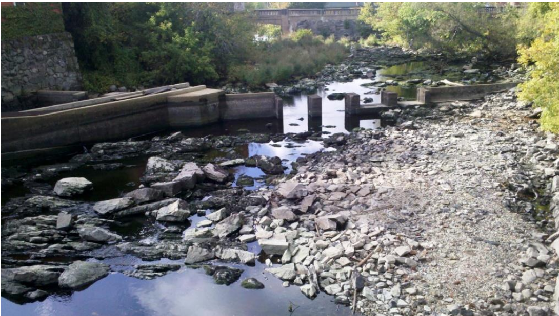
View of fish passage on left and concrete weir in center, facing N
