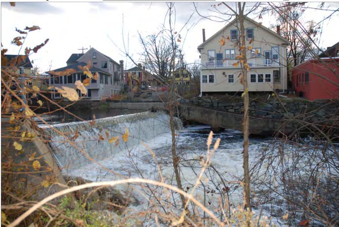
Photo # 7 Description: View of dam and fish passage from east bank of Exeter River Roll and Frame # OR Digital file name: EXE0043_07 Direction: W
