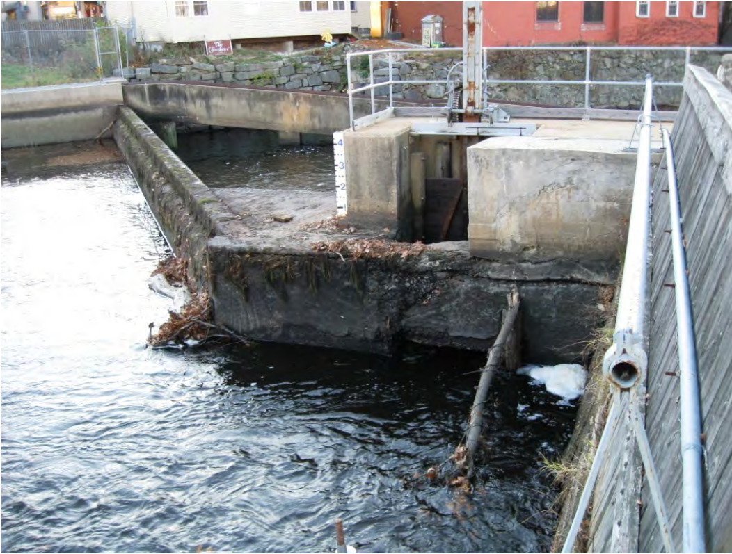
View of dam, fish passage (top center), portion of penstock baffle wall (far right), and low-level gate (center). Facing W.
