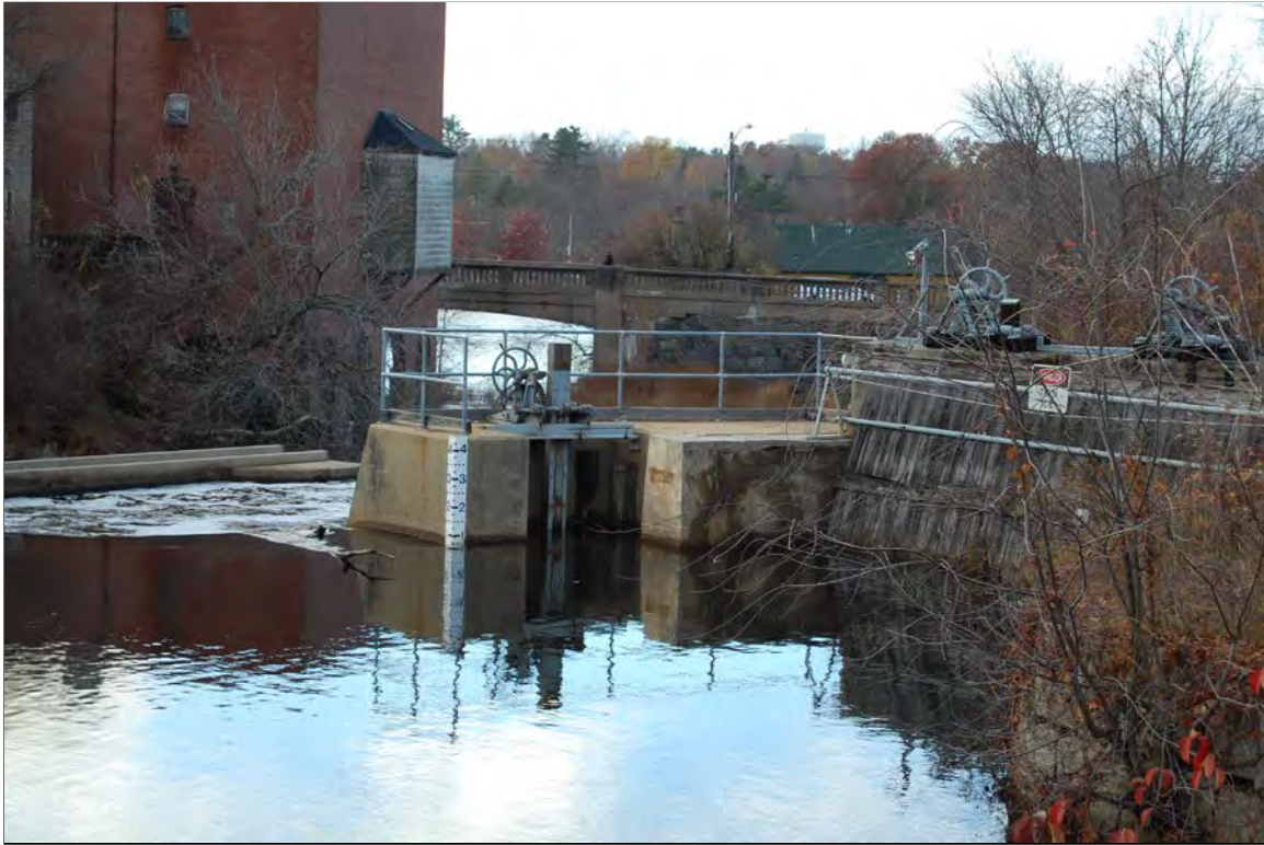
Photo # 4 Description: Low-level gate (center) and penstock baffle wall (right) Roll and Frame # OR Digital file name: EXE0043_04 Direction: NW
