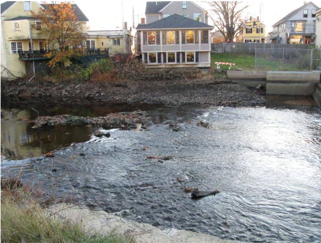
View of ledge outcrops in area just upstream of dam (dam is on far right), facing W
