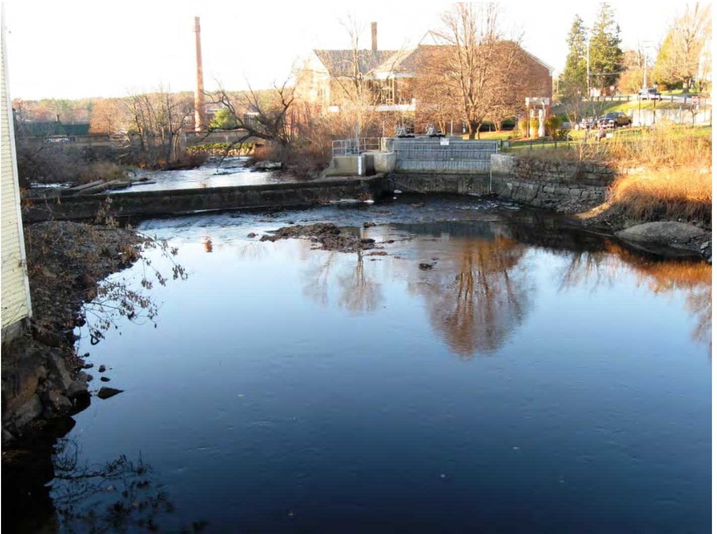
View of dam from High Street Bridge, facing N. Dam is shown in center, with penstock baffle (wood) wall and low-level gate on right hand side of photograph.
