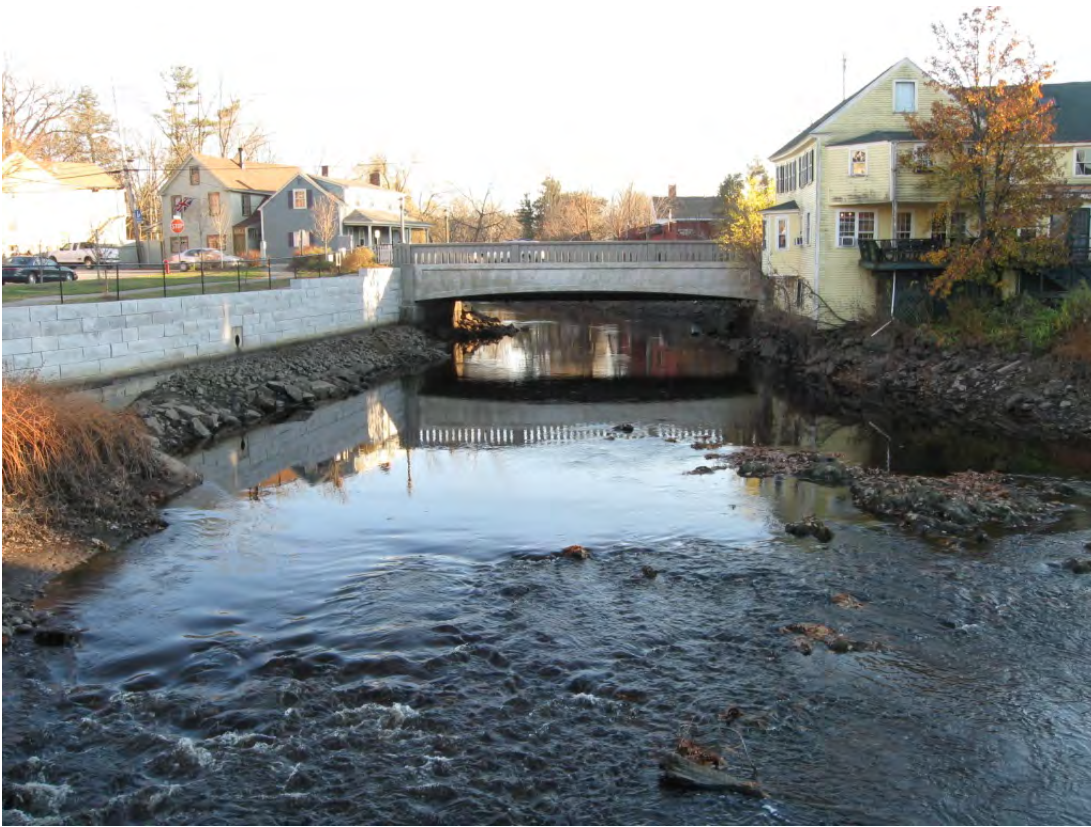
View of ledge outcrops just upstream of dam, facing S towards High Street bridge
