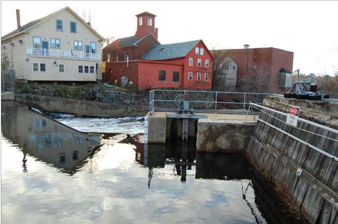
Photo # 3 Description: Fish passage (left) and penstock baffle wall (right) and low-level gate (center) Roll and Frame # OR Digital file name: EXE0043_03 Direction: NW
