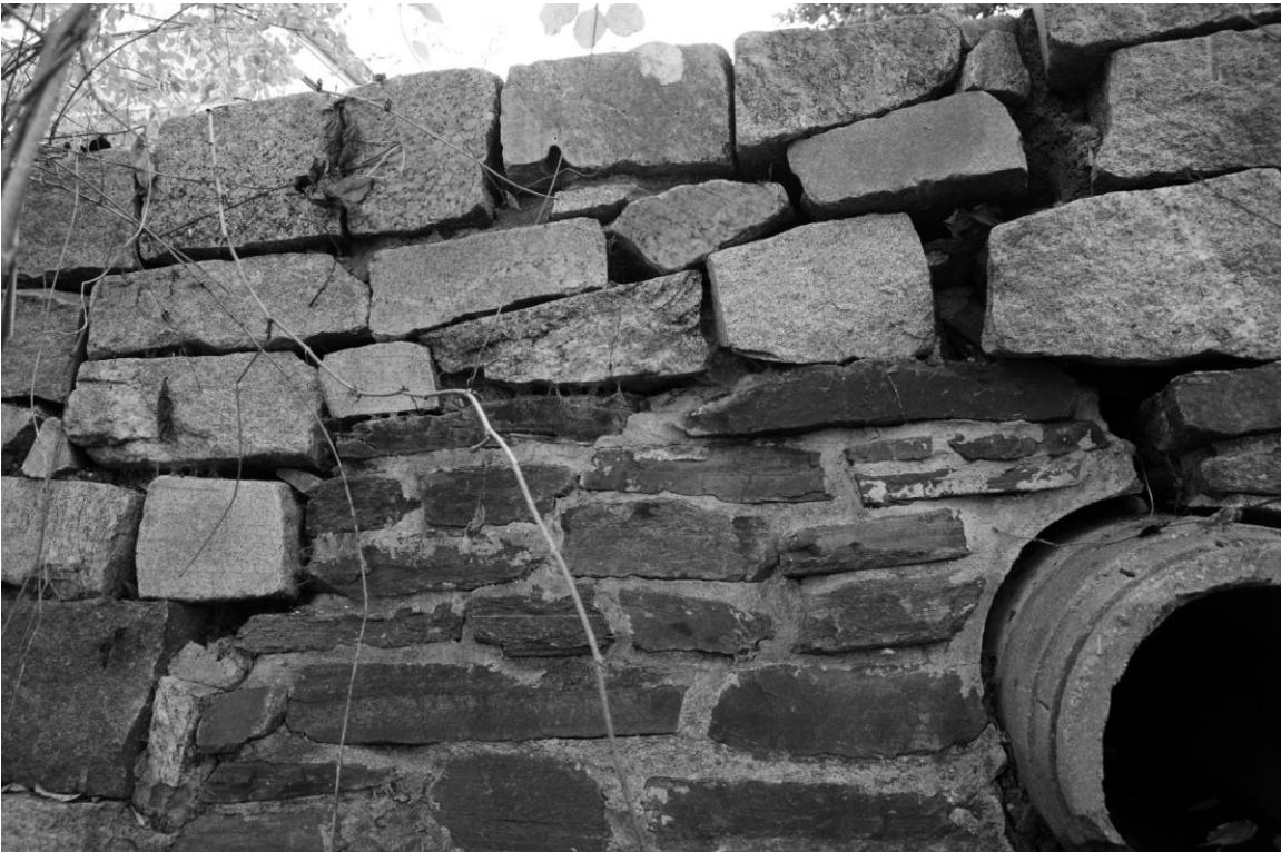
Photo 106 description: Wall No. 5, downhill face, showing two types of stone with culvert.
