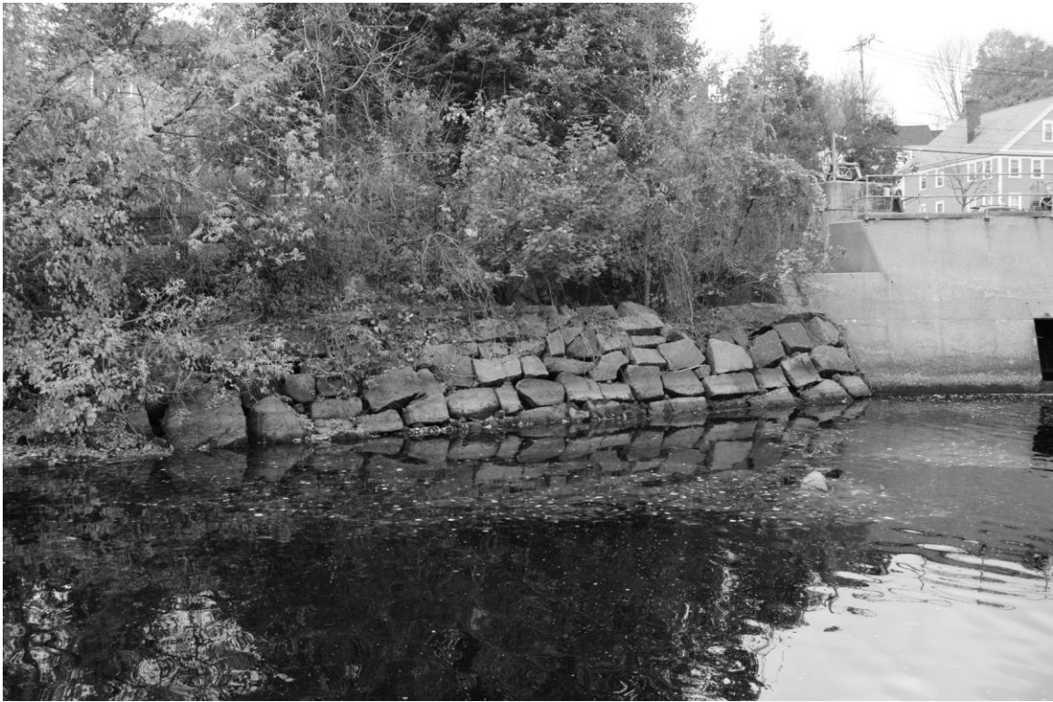
Photo 103 description: View of rip-rap slope downstream of dam headworks (Wall No. 3). Roll: _____ Frame: _____ Direction: NE Date taken: 10/2014 Negative stored: _____
