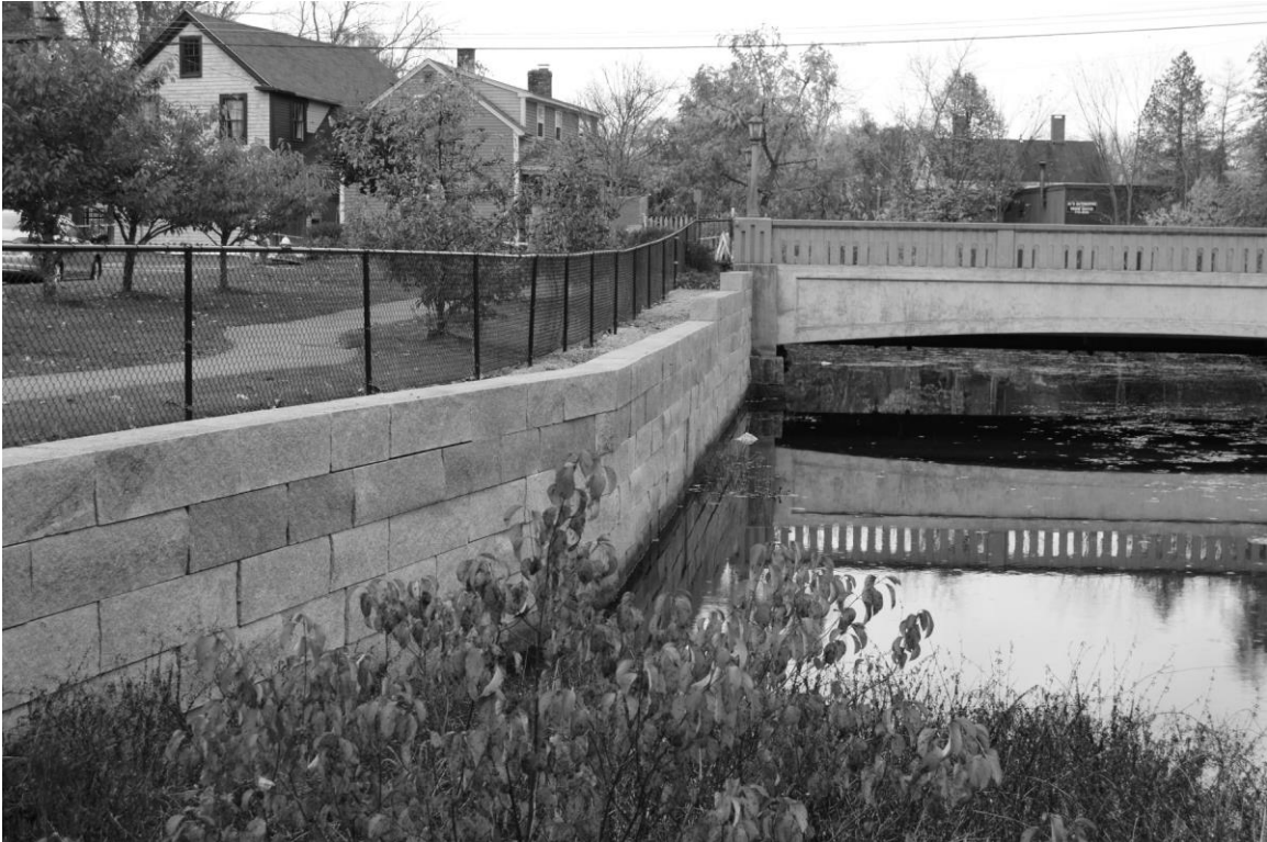
Photo 99 description: New granite wall along east bank (Wall No. 1), with Great Bridge in background. Roll: _____ Frame: _____ Direction: S Date taken: 10/2014 Negative stored: _____
