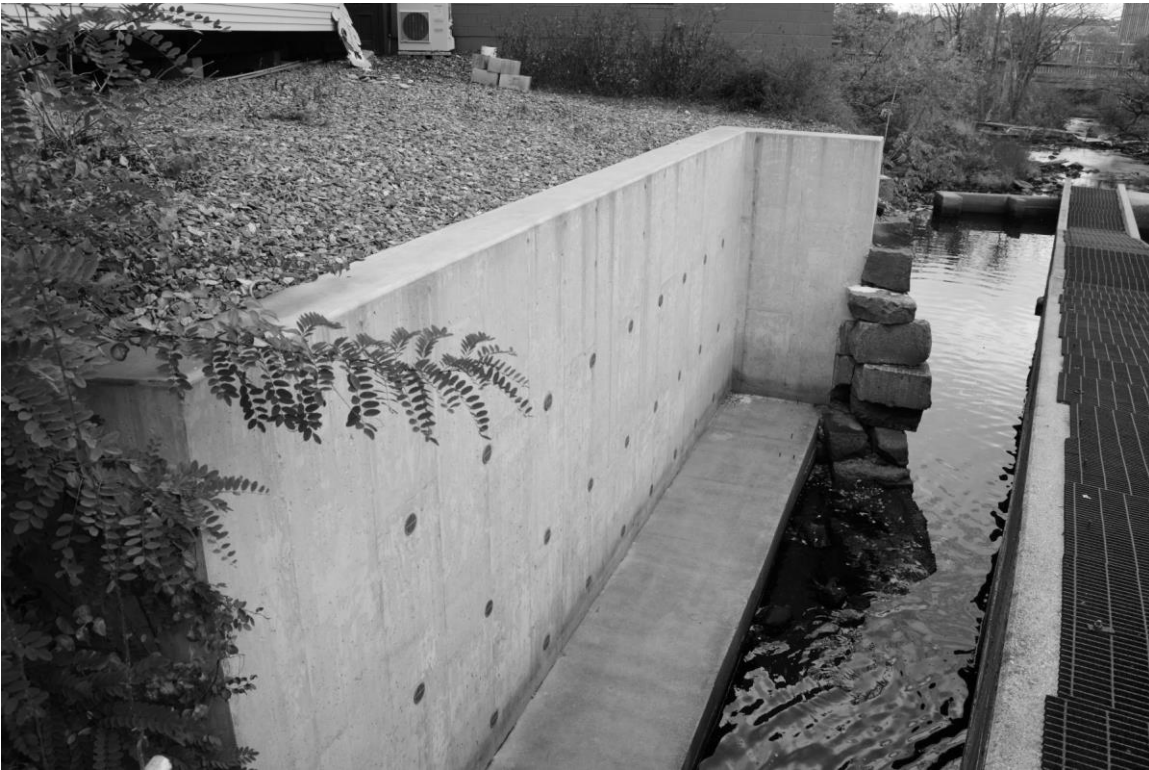
Photo 111 description: View of concrete wall at 27-31 Water Street (Wall No. 7), showing footing.
