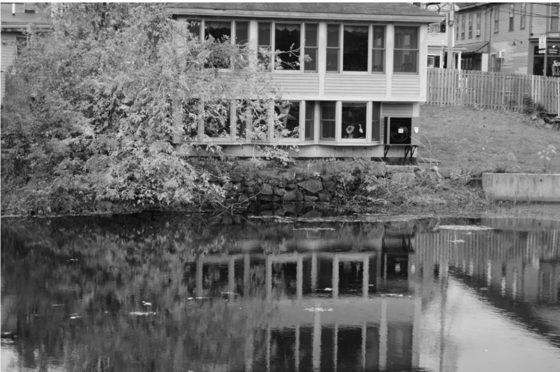
Photo 114 description: Foundation wall at 11 Water Street (Wall No. 9). Roll: _____ Frame: _____ Direction: SW Date taken: 10/2014 Negative stored: _____
