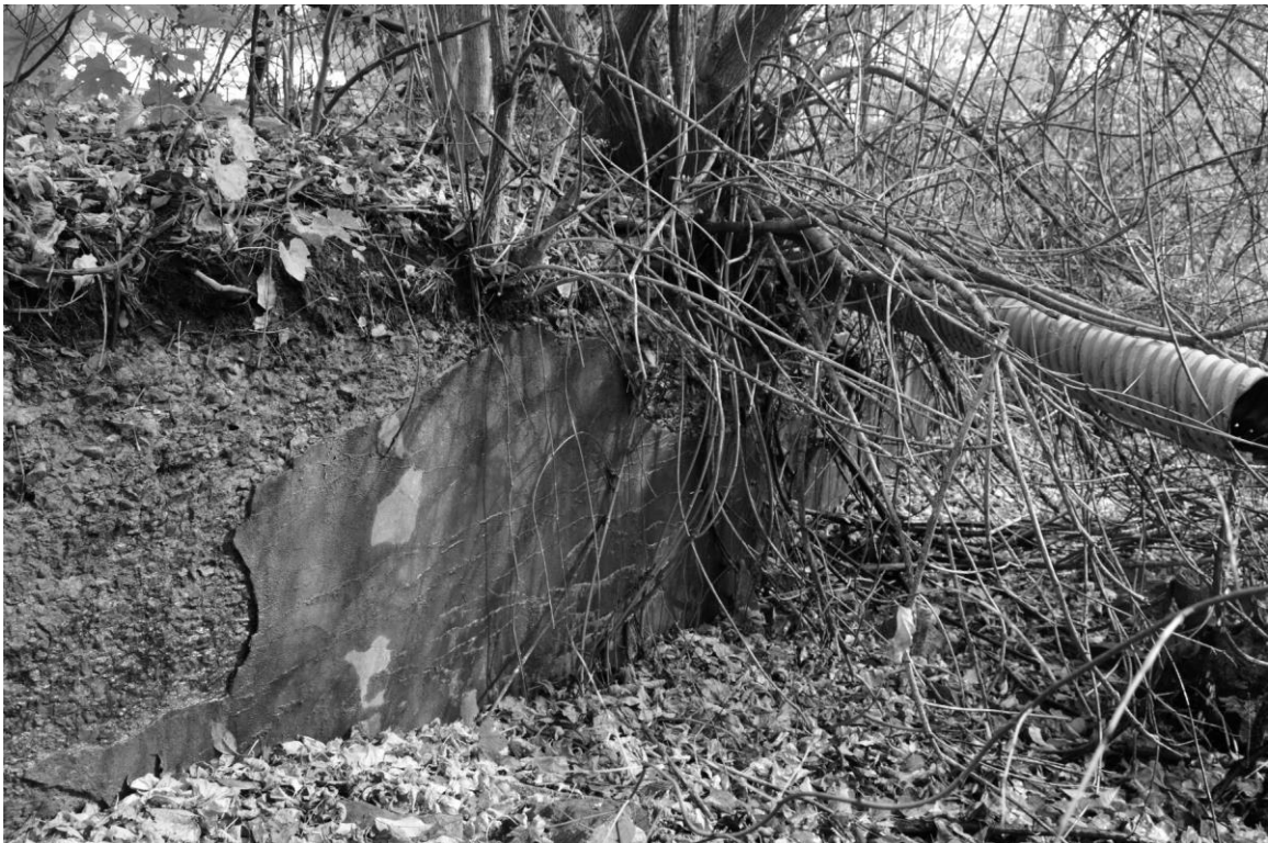
Photo 104 description: View of Wall No. 4, showing deterioration and culvert pipe. Roll: _____ Frame: _____ Direction: NE Date taken: 10/2014 Negative stored: _____
