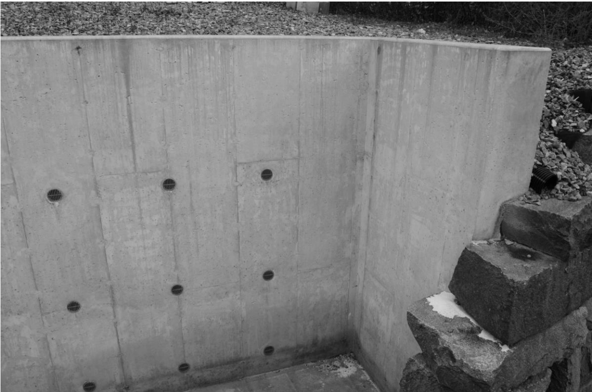
Photo 110 description: View of new concrete wall behind 27-31 Water Street (Wall No. 7). Roll: _____ Frame: _____ Direction: SW Date taken: 10/2014 Negative stored: _____
