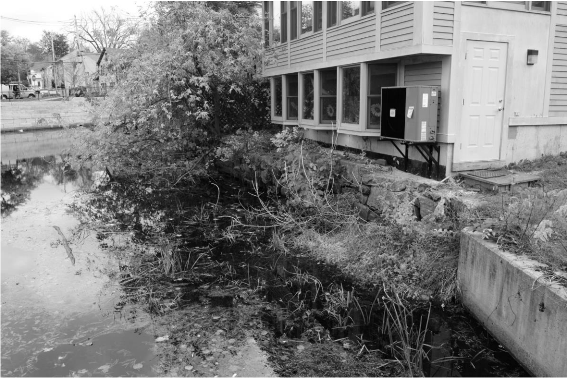
Photo 113 description: Foundation wall at 11 Water Street (Wall No. 9), with portion of Wall No. 8. Roll: _____ Frame: _____ Direction: SW Date taken: 10/2014 Negative stored: _____
