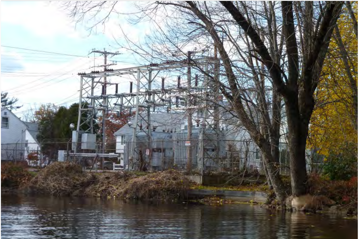
Photo 83 description: View of electric transformer station on River Street from Exeter River
