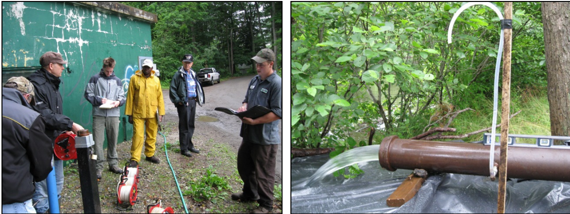
Preparing for Pumping Test Observations (July 2009) and Gilman Pump Discharge Line
