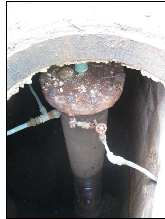
Manifold Pipe in Collector Well
