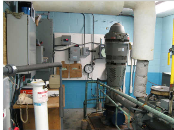
Lary Lane Well Pump and Controls
