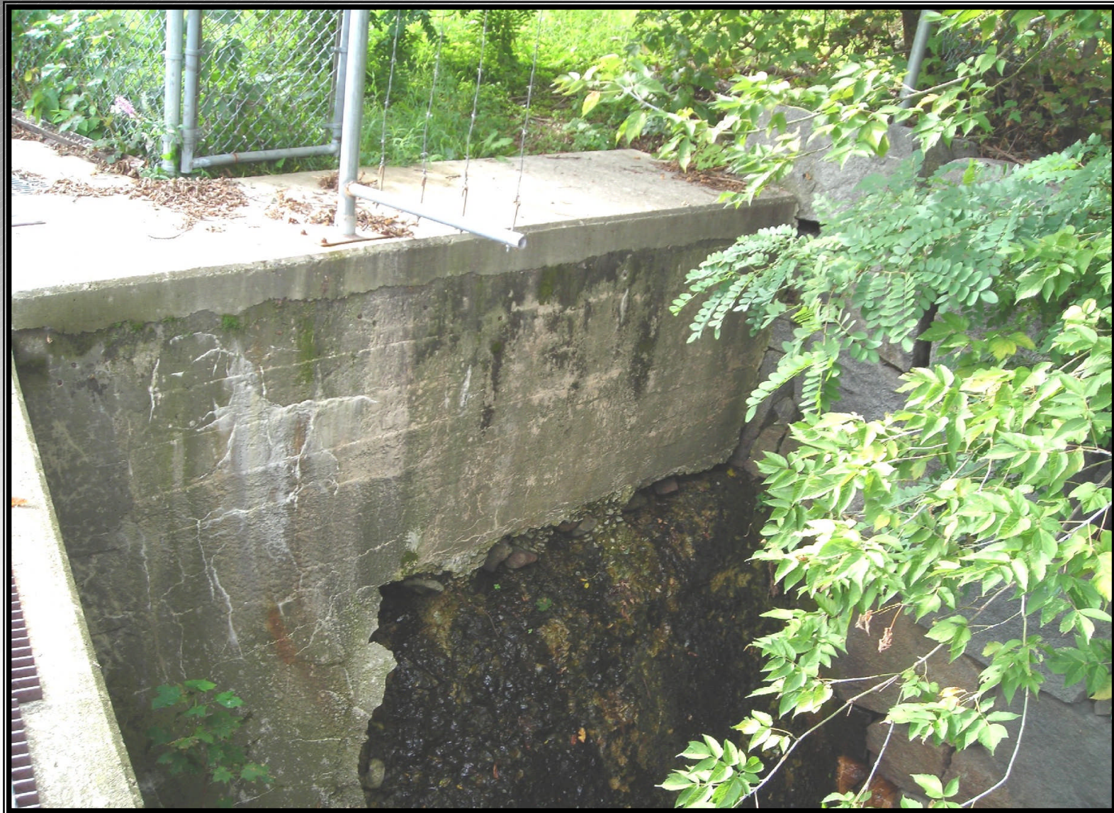
Spalled area west of fish ladder
