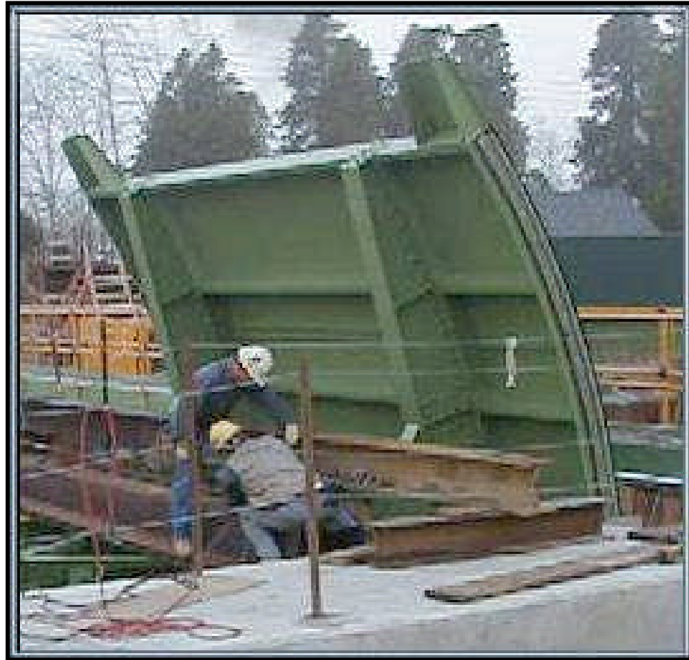
“Tainter” Style Discharge Gate
