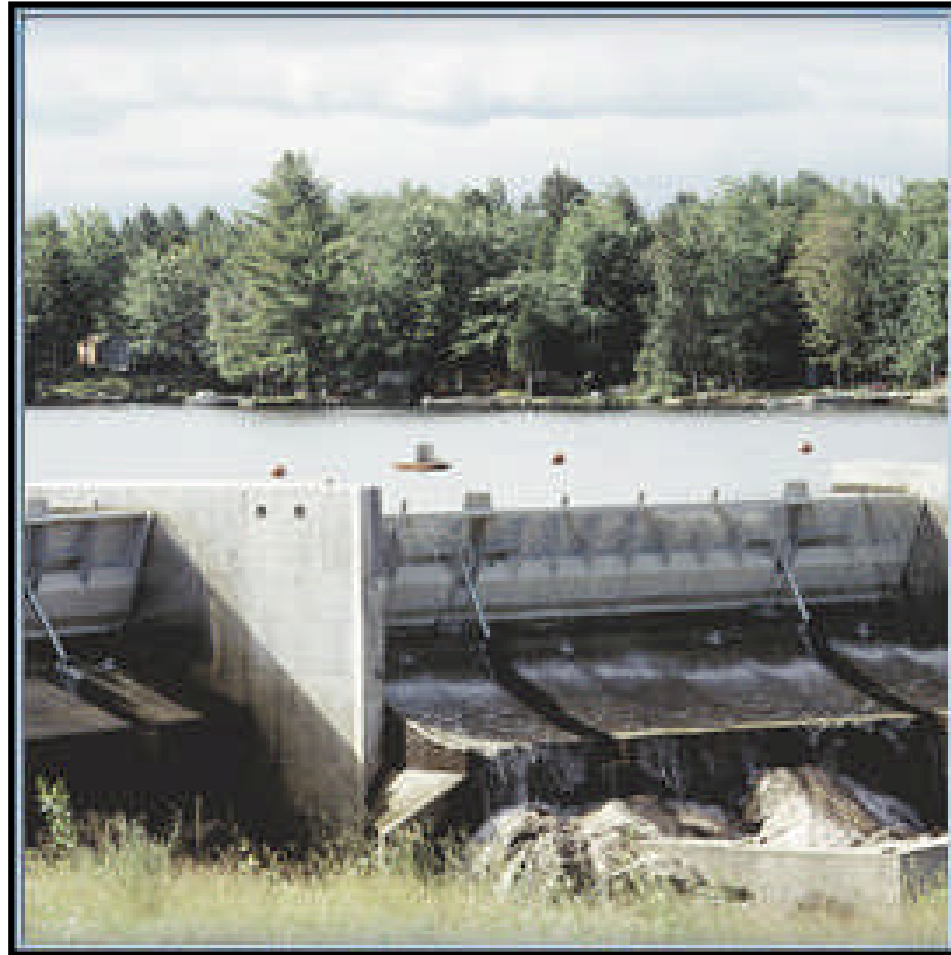
Crest Gate Operated from Below
