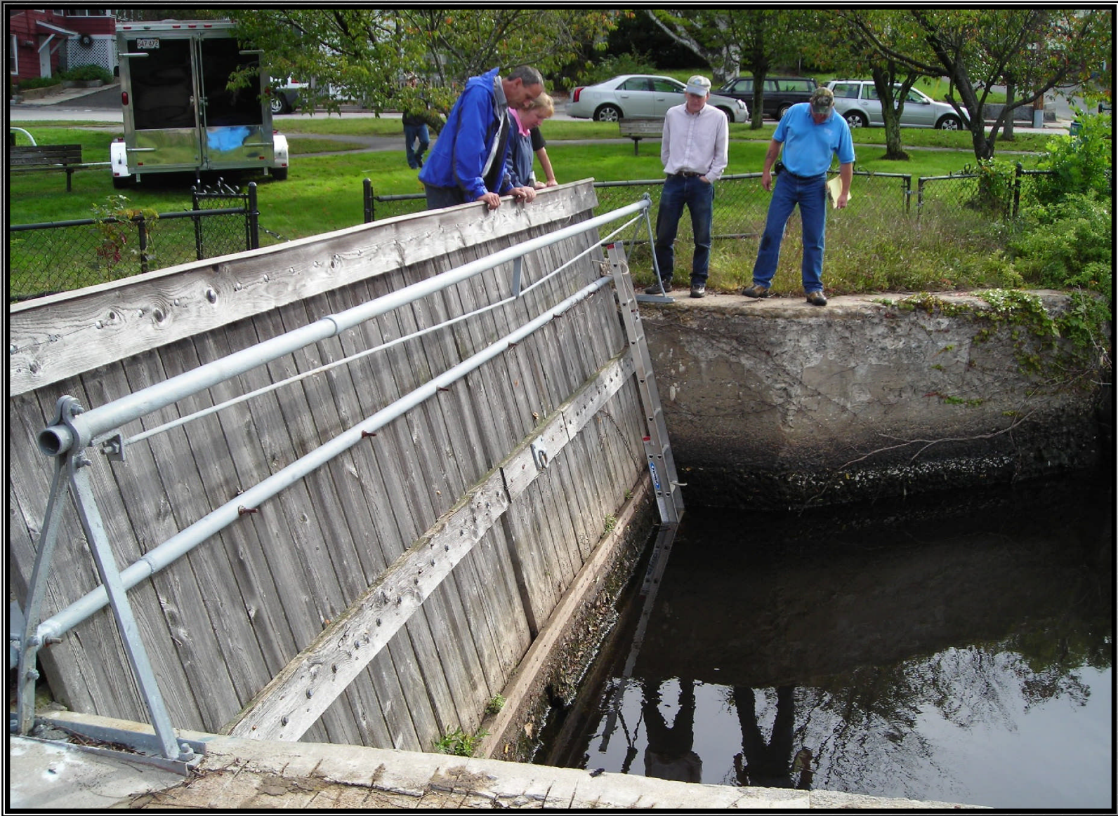
Great Dam Penstock Baffle
