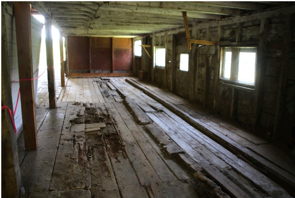
Photo 41) South aisle and whitewashed animal tie up area, showing deteriorated floor condition
