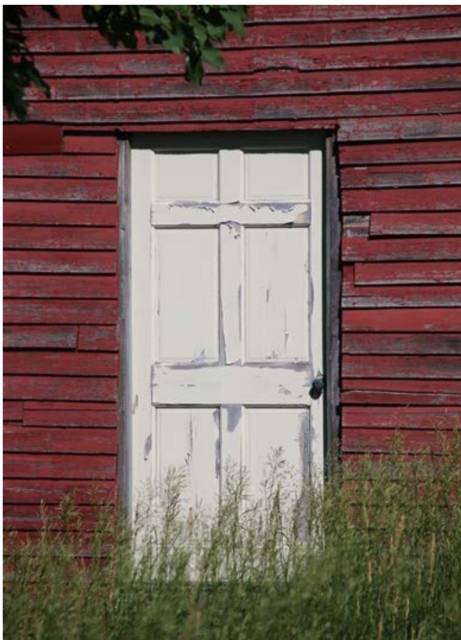
Photo 22) East elevation, south doorway, showing 1960s residential door in former sliding door opening Direction: W
