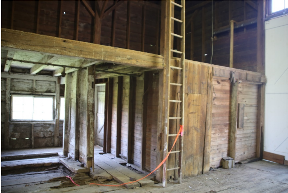
Photo 37) Southwest corner milk room, ladder to hayloft, animal tie up area at left with deteriorated flooring at stanchion Direction: SW
