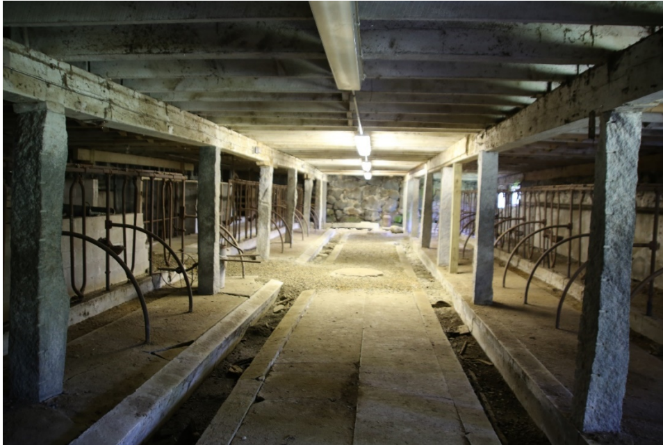
Photo 52) Basement milking area, milking stanchions and central aisle with granite support columns, looking east. New drainage catch basin in center aisle.
