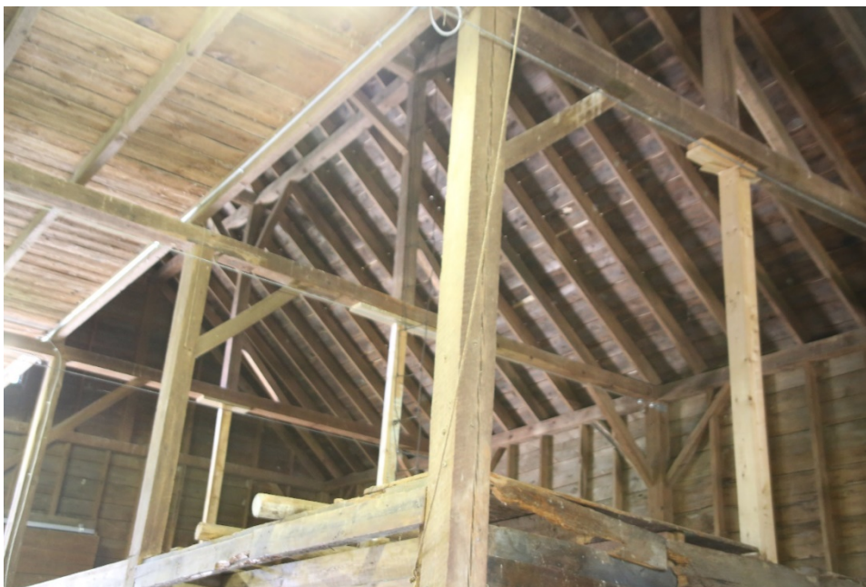
Photo 28) Detail of framing along central drive bay, showing tie beams and temporary supports beneath purlin posts, adjacent to the hayloft above Direction: NW
