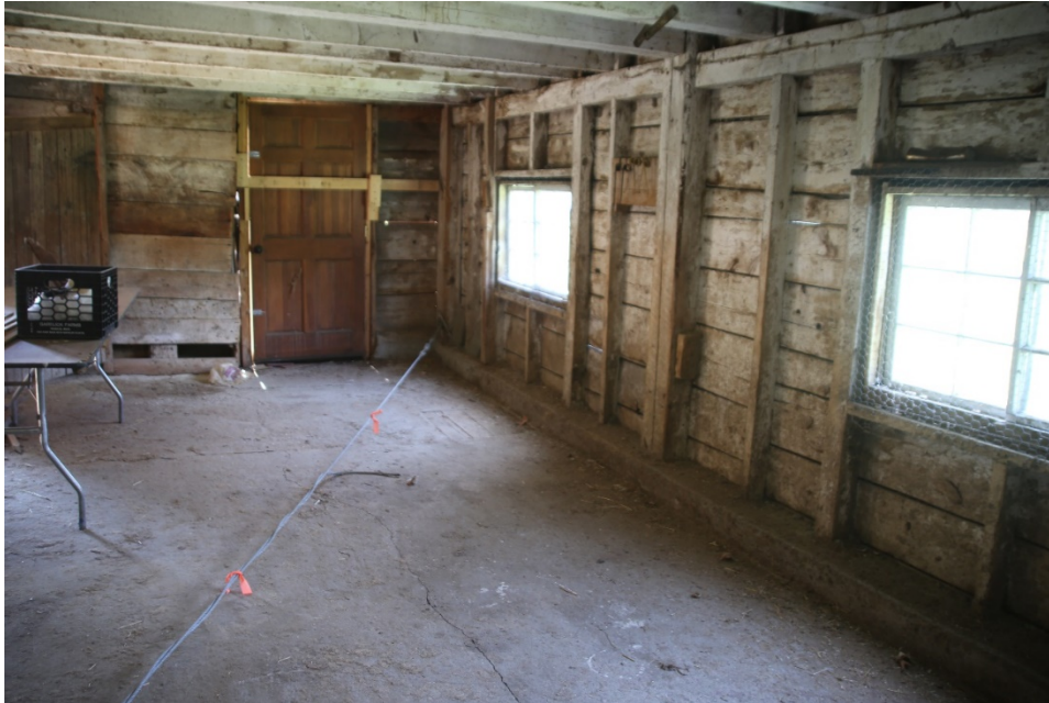
Photo 42) Southeast room, privy area with whitewashed walls and 1960s residential door in former sliding doorway. Assume cable introduced to maintain integrity of corner posts while foundation was being repaired.
