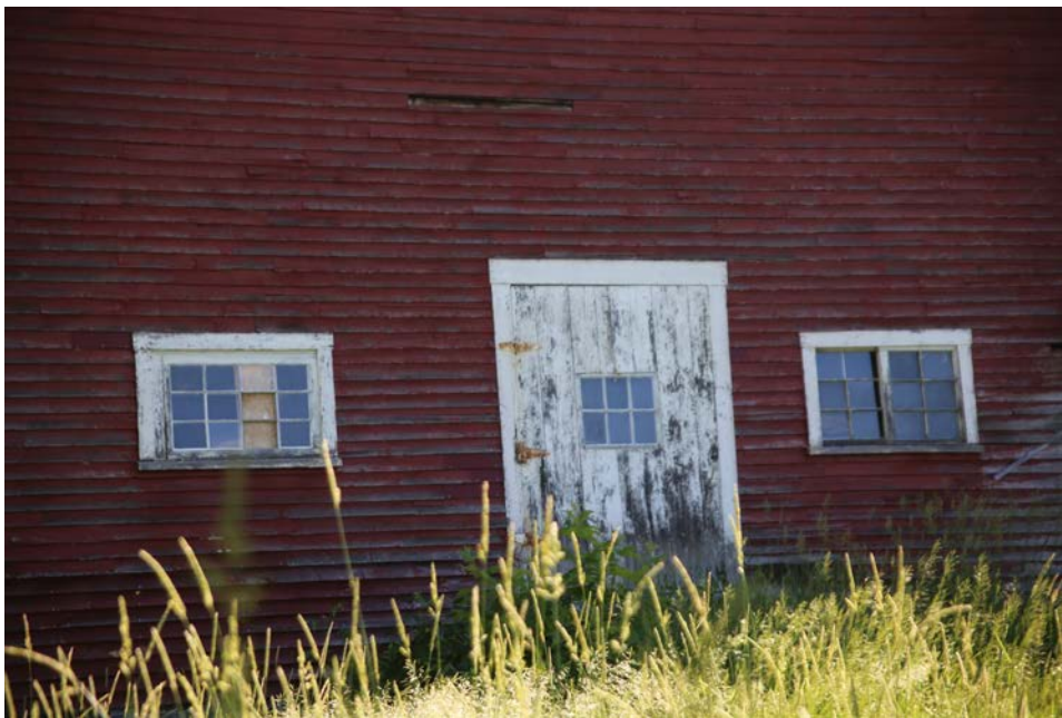
Photo 14) South elevation, cow door at top of ramp, showing window conditions Direction: NNE
