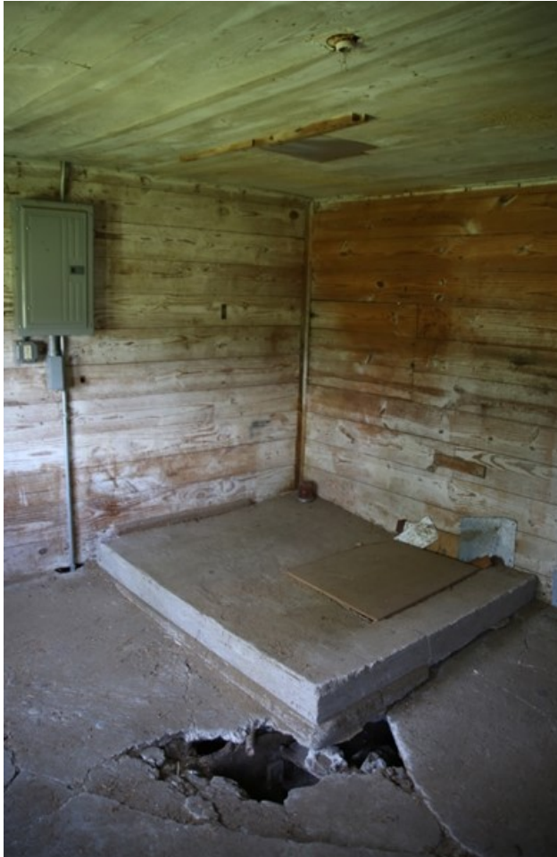
Photo 38) Main floor milk room later grain room, southwest corner, showing yellow pine walls and ceiling boards, deteriorated concrete floor, and upgraded electrical system Direction: NW
