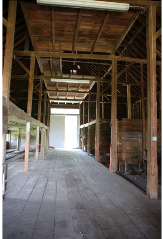
Photo 26) Central drive bay, looking west, with haymow area on right, calfpen area on left, and hayloft above Direction: W
