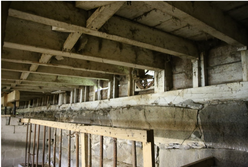
Photo 59) East end of North foundation wall and sill, exhaust fan Direction: NW
