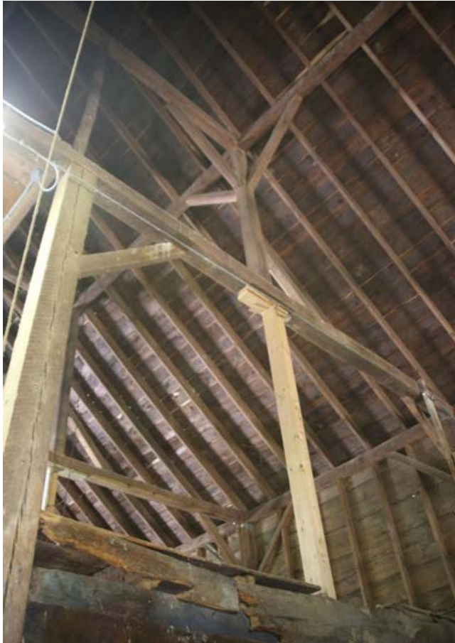
Photo 27) Detail of wall and roof framing showing temporary post beneath the purlin posts to support the tie beam, cables visible. Direction: NW
