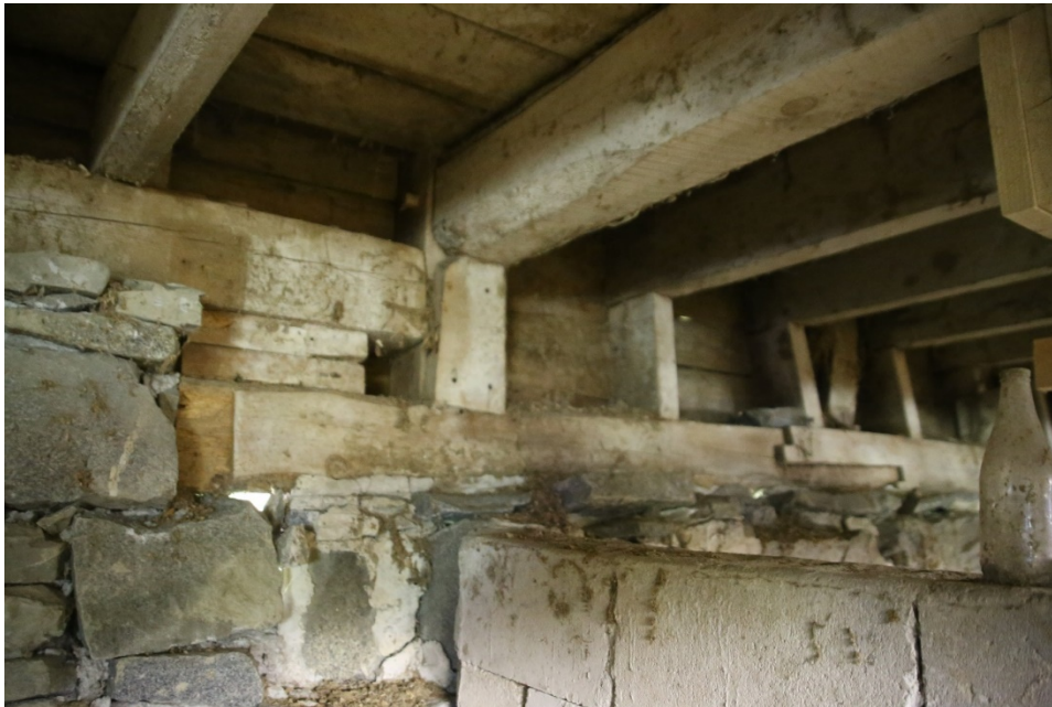
Photo 57) North foundation wall and sill, reconstructed area to left Direction: NNE
