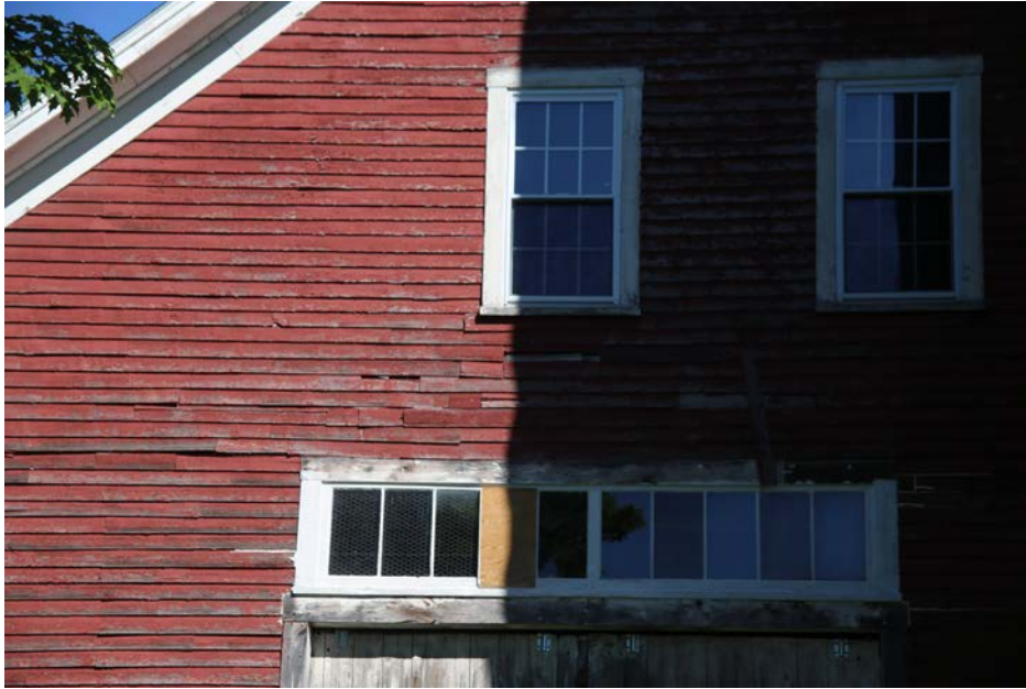
Photo 21) East elevation, showing clapboard condition and broken transom lights, vinyl replacement windows in gable Direction: W
