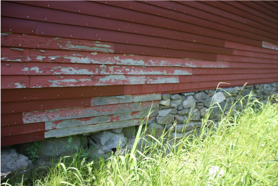
Photo 17) North elevation, showing clapboard condition and foundation walls. Foundation wall repair from 2004 seen at right, failing foundation wall in need of repair at left. Direction: SE
