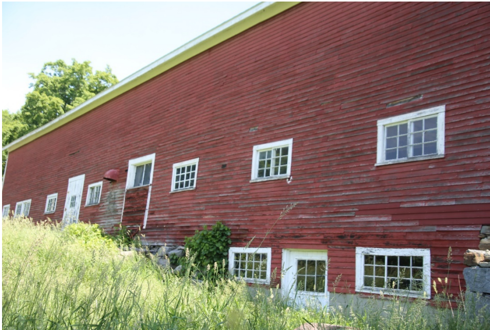
Photo 13) South elevation, showing variety of windows and condition of clapboards Direction: WNW
