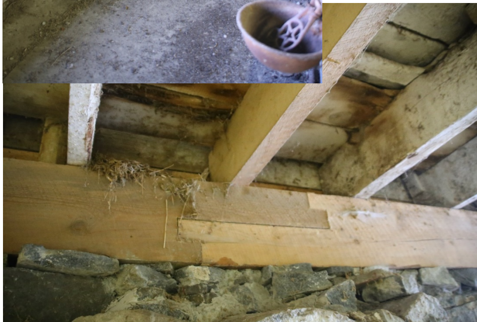
Photo 63) South foundation wall, new sill, and floor joists, sections replaced in 2006 Direction: S
