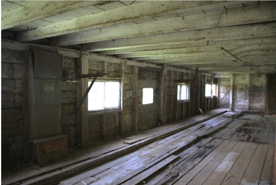
Photo 40) South aisle and whitewashed animal tie up area, outline of original gutter, showing deteriorated floor condition
