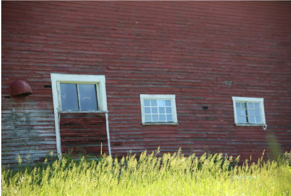
Photo 15) South elevation, infilled door with clapboards and window sash, showing window conditions and ventilator hood at left
