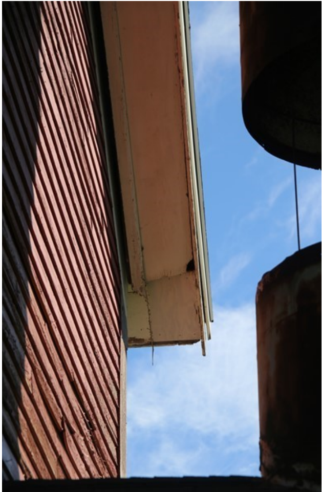
Photo 23) East elevation, north raking eave, showing separation of molding from the building Direction: N
