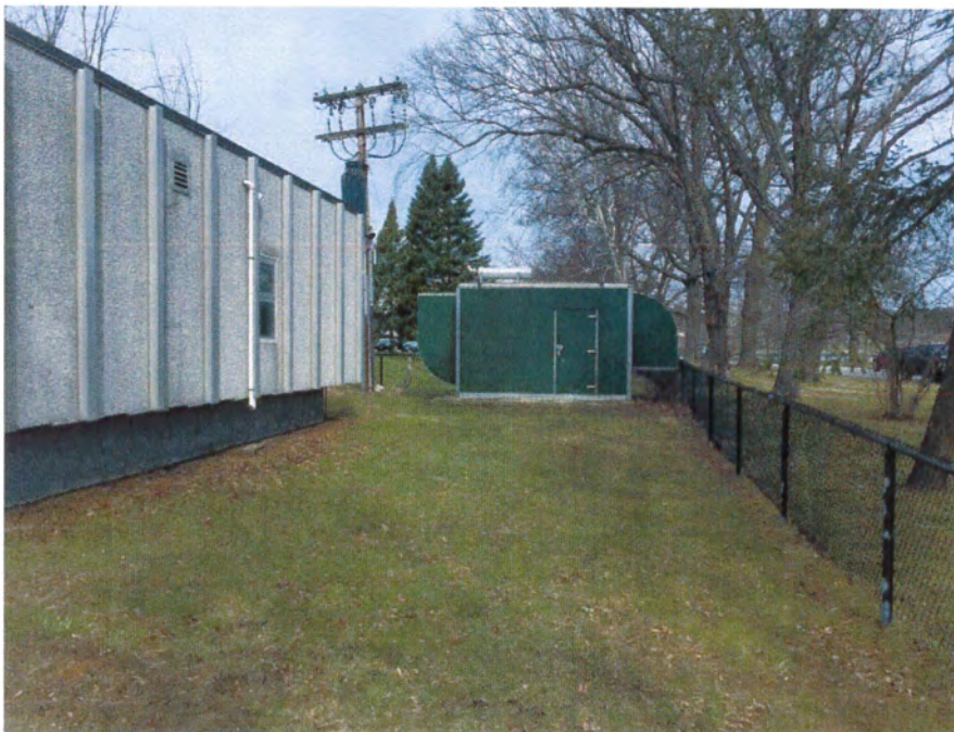
Main PS & Generator
