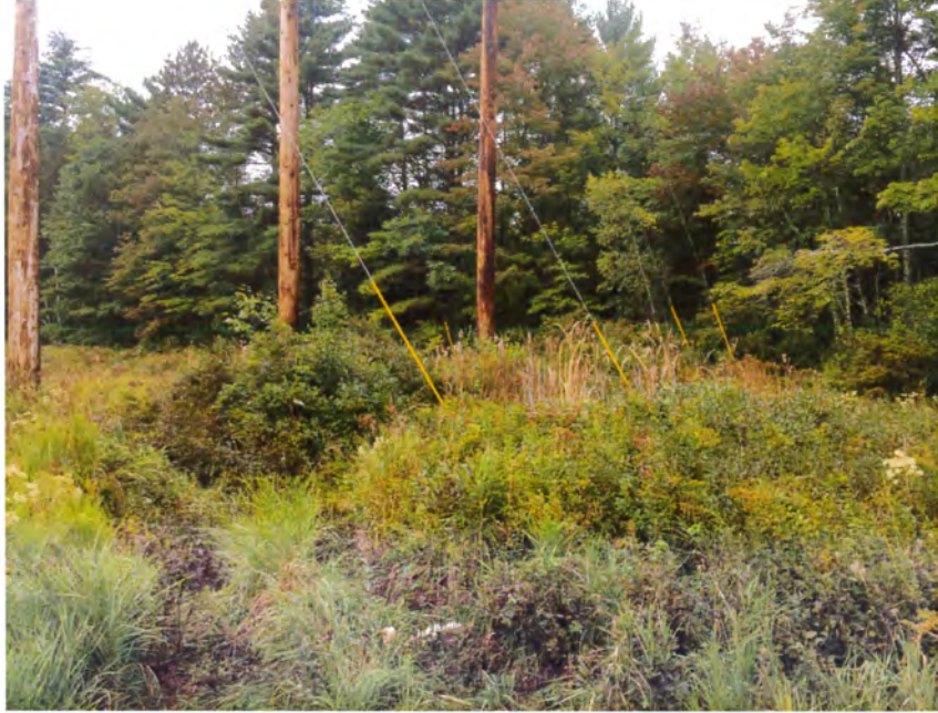
Photograph No. 7: Looking westerly at A126 Structure 186 guy wires to be replaced.
