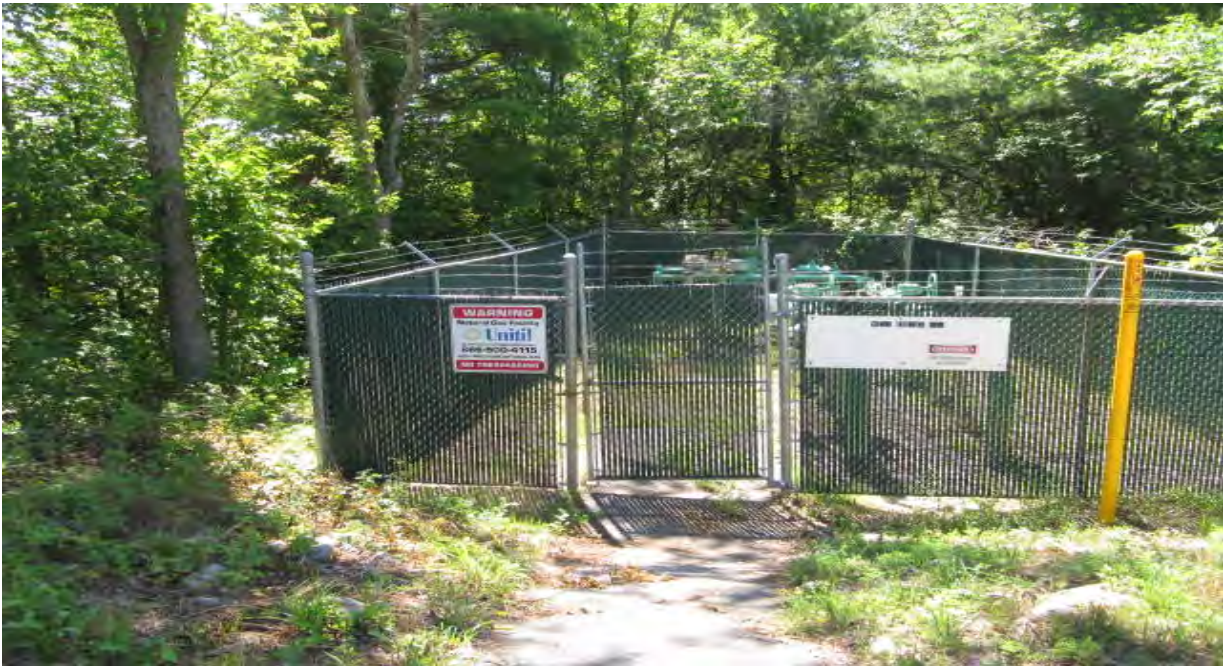
Photo S-2. Unitil gas valve located along the western side of Wetland S.
