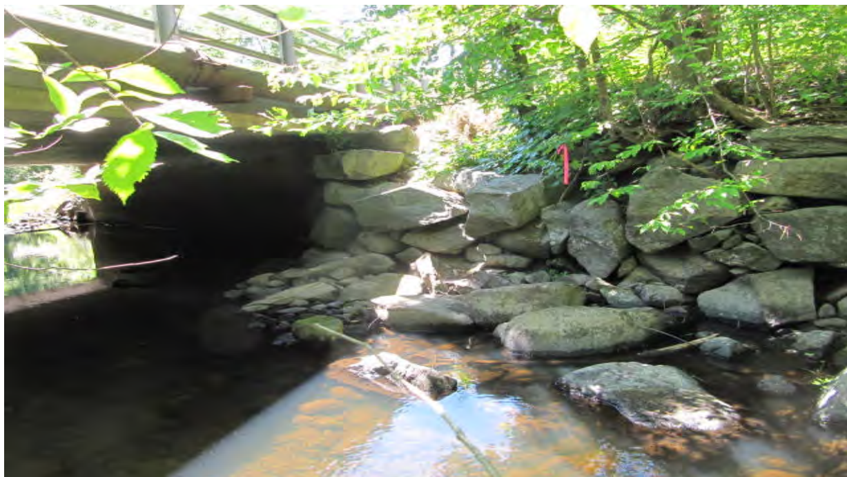
Photo T-3. Heavily riprapped Bank of Little River along the northwestern side of Route 111. This area was delineated with flags V1 to V4.
