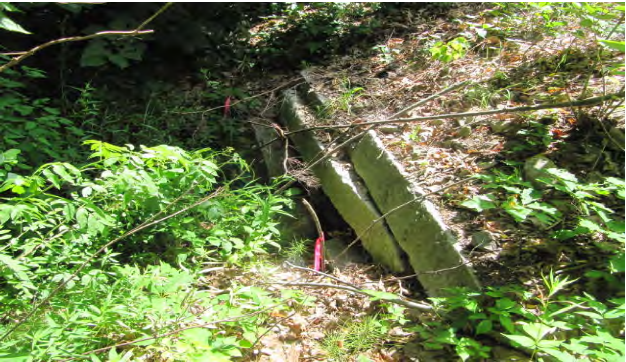
Photo H-2. View of granite slabs used as a headwall over 16" cp along north side of Route 111.
