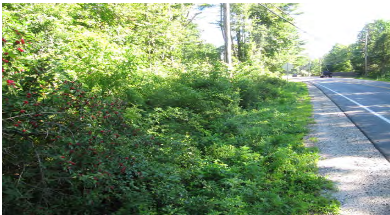
Photo T-4. Top of Bank of Little River along the northwestern side of Route 111. The Bank drops off almost vertically just off the road into the river.
