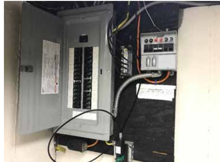
Photo 12: Breaker panel located in the basement.
