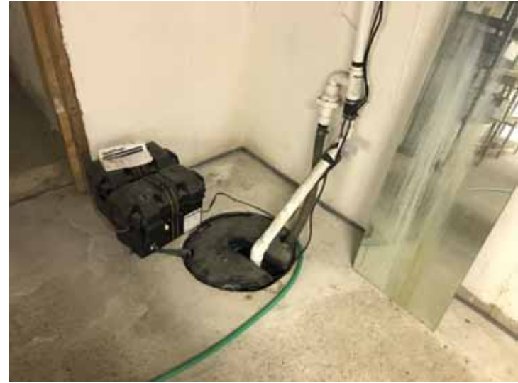
Photo 10: Sump located in the basement.
