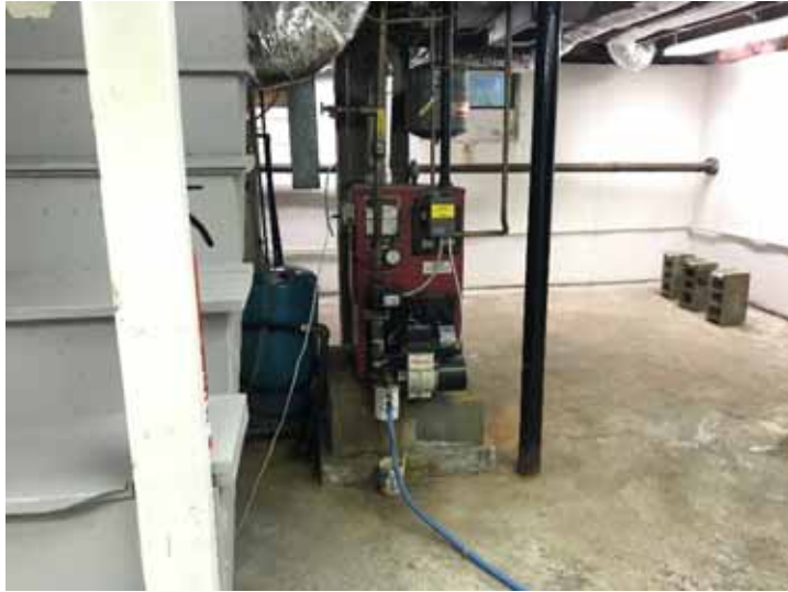
Photo 13: Boiler and pressure tank located in the basement, facing south.
