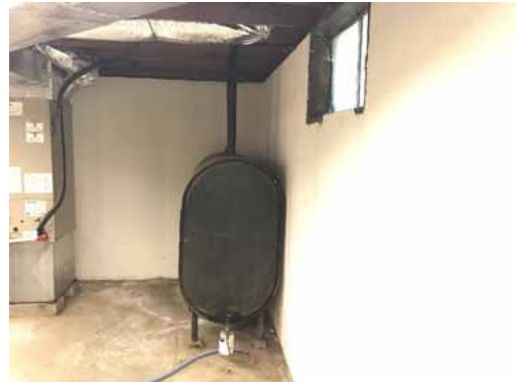
Photo 8: AST located at the northwest corner of the basement, facing west.
