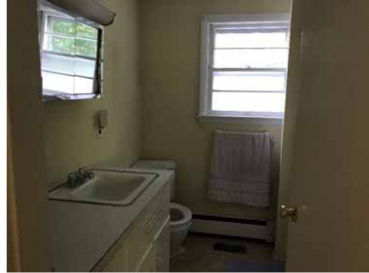
Photo 6: First floor bathroom located on the south side of the residence immediately west of the kitchen, facing south.
