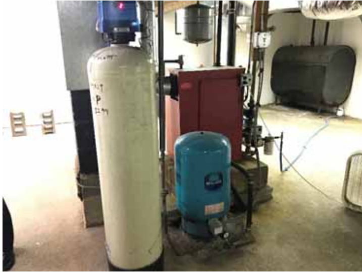
Photo 9: Pressure tank and water softener located in the basement, with the boiler directly behind, facing northwest.
