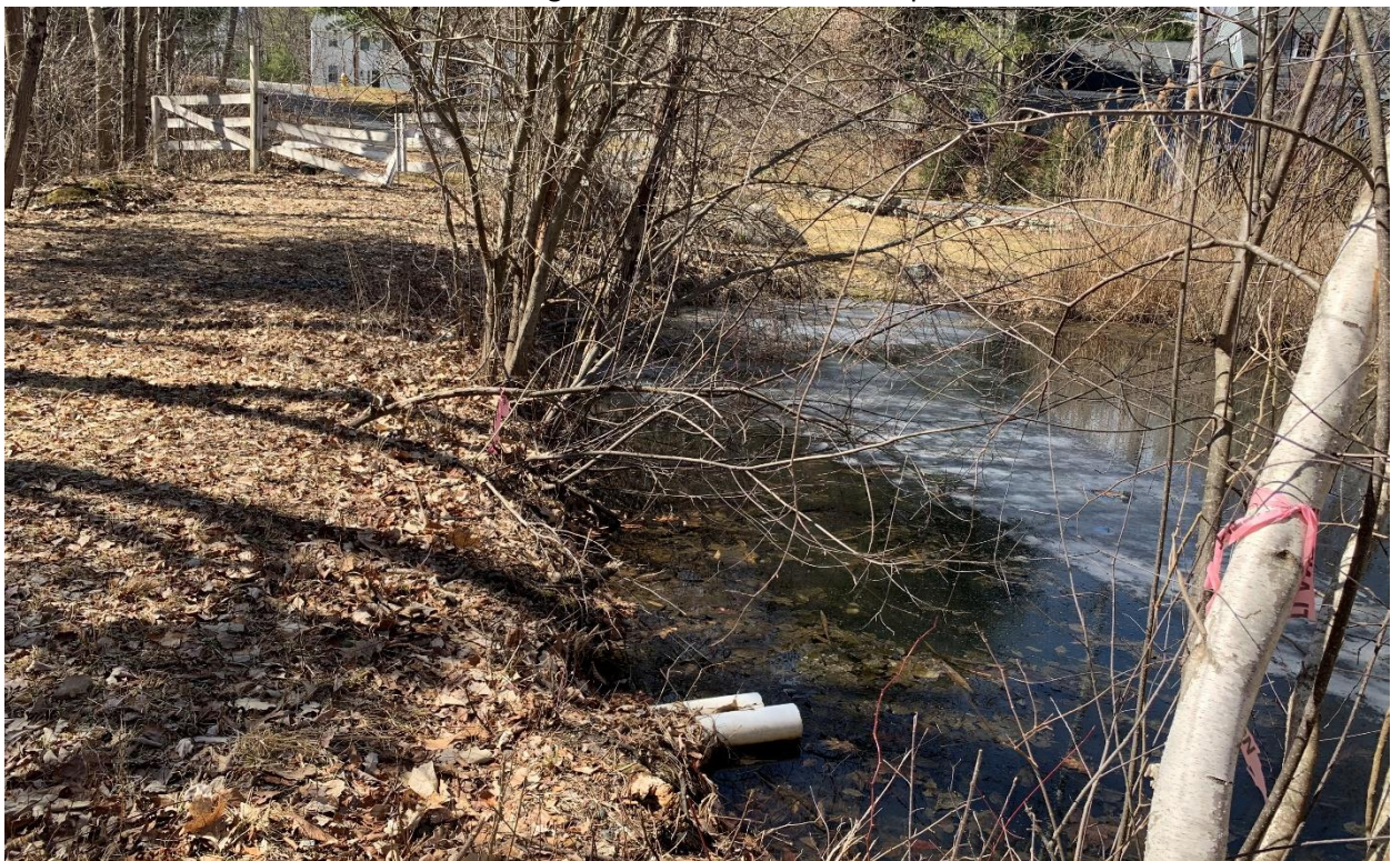
Photo #4: Looking to the west at wetland impact #2 to the man- made pond and the outlet pipes that will be replaced.
