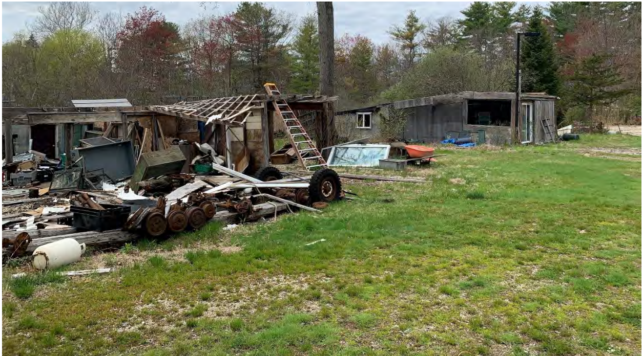
Photo #2: Looking to the north at the deteriorating building and structures that extend into the wetlands.
