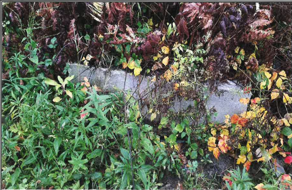
Photograph 13- View of concrete in GH Area. (StoneHill, October 11, 2017)
