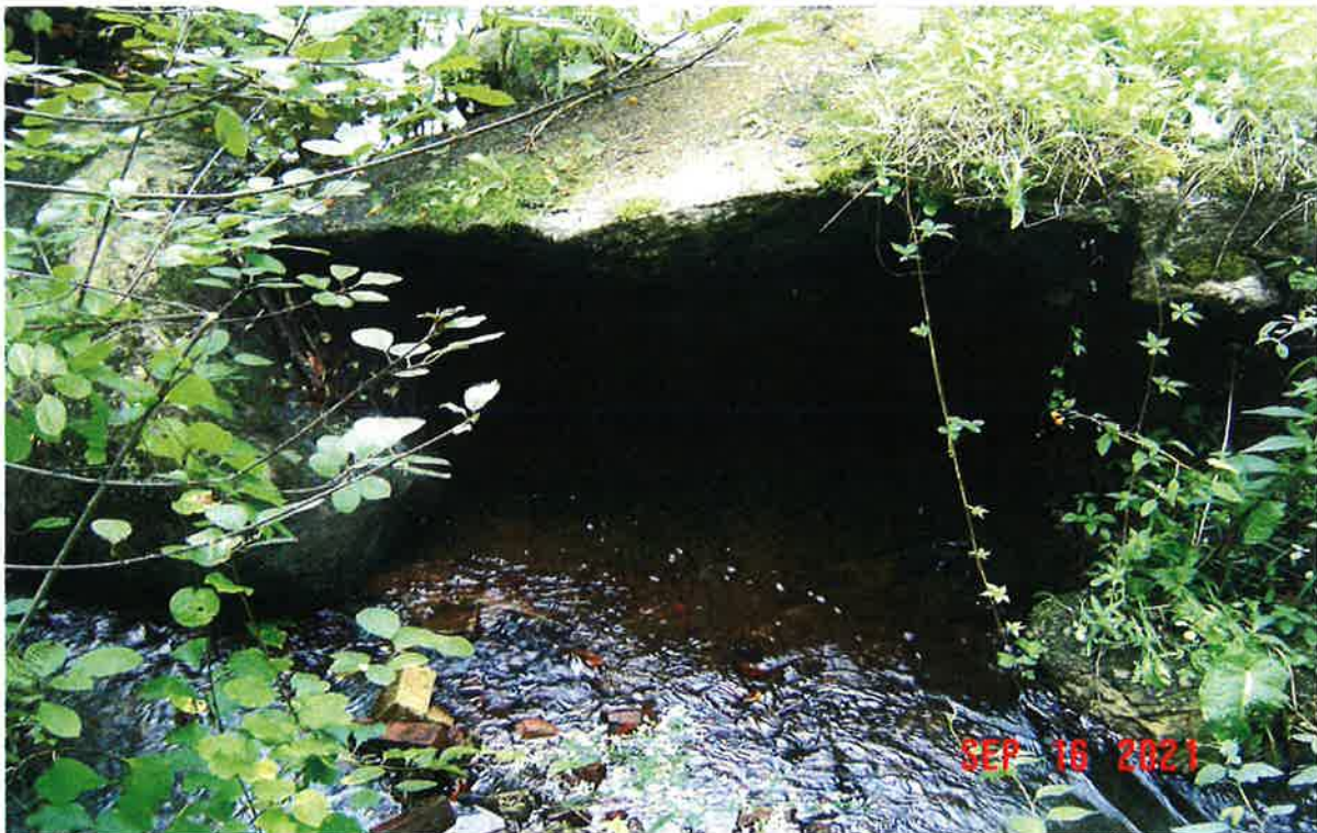
Image 28 – Looking at breach in concrete weir and general location of proposed repair and installation of fish ramp. (This is just left of weir as shown in image 6.) Refer to Figure 1. ©Jacobs2021
