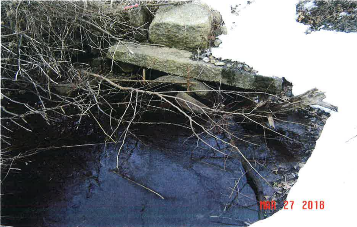
Image 23 – Looking at upstream end of culvert D4. Note culvert is almost running full; compare to image 21. Refer to Figure 4. ©Jacobs2018
