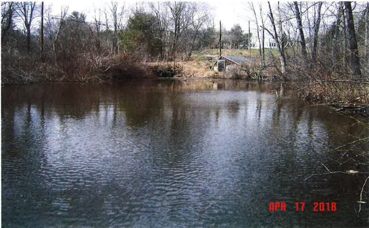
Image 20 – Looking north (upstream) at culvert D4 and Oak Street Extension (in the background) from the concrete weir. Note pump house on right. Refer to Figure 1. ©Jacobs2018
