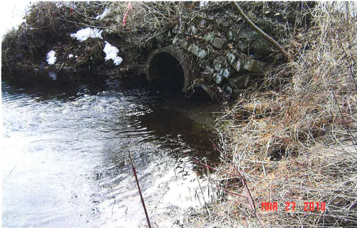
Image 21 – Looking southwesterly at the downstream end of culvert D4 from the pump house. Refer to Figure 4. ©Jacobs2018
