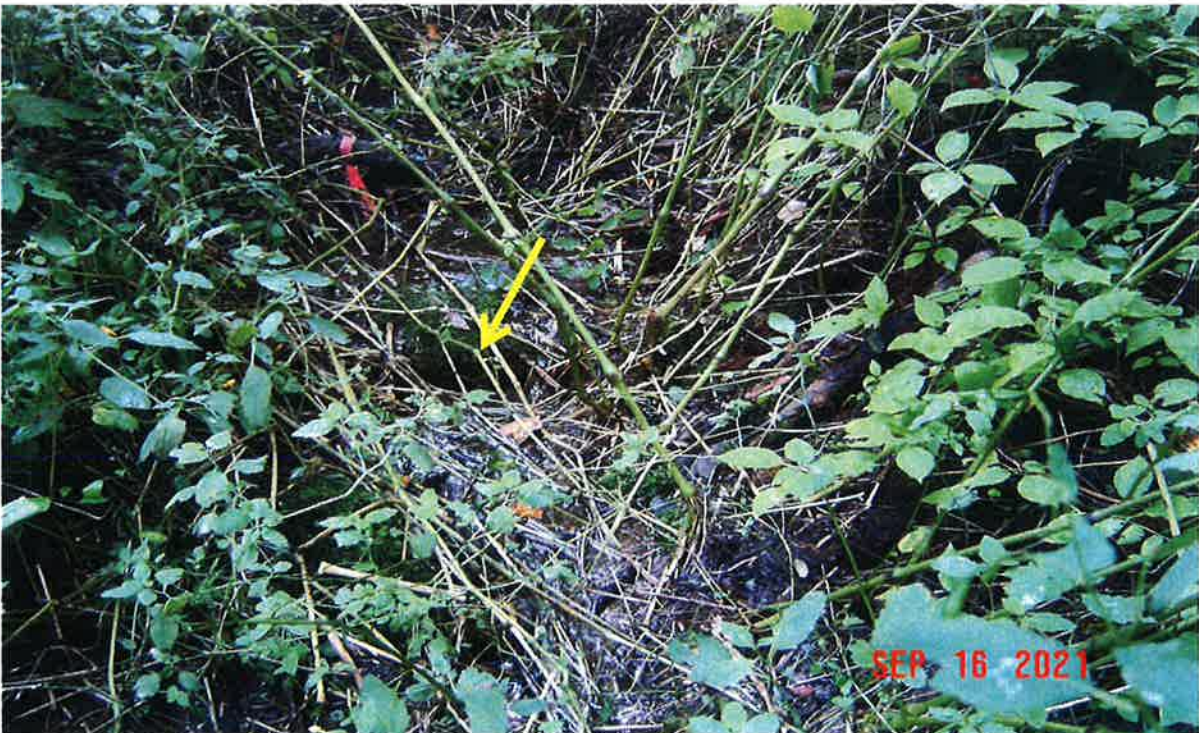
Image 24 – Looking at downstream / plugged end of culvert D2 (yellow arrow). 142 SF of impact to Wetland J proposed here for replacement of culvert D2. Refer to Figure 3. Note pink wet flag. ©Jacobs2021
