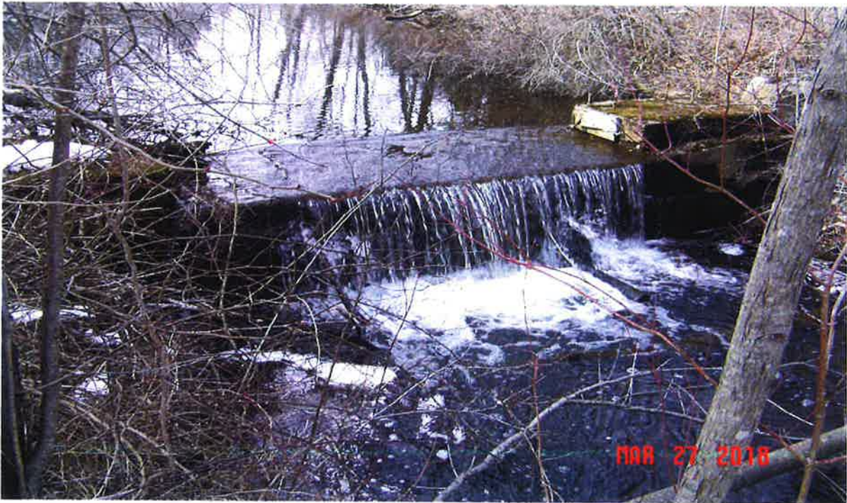
Image 6 – Looking northwesterly at the concrete weir. Note the pipe on lower right in the foreground and flooded man-made pond in the background. Refer to Figure 1. ©Jacobs2018
