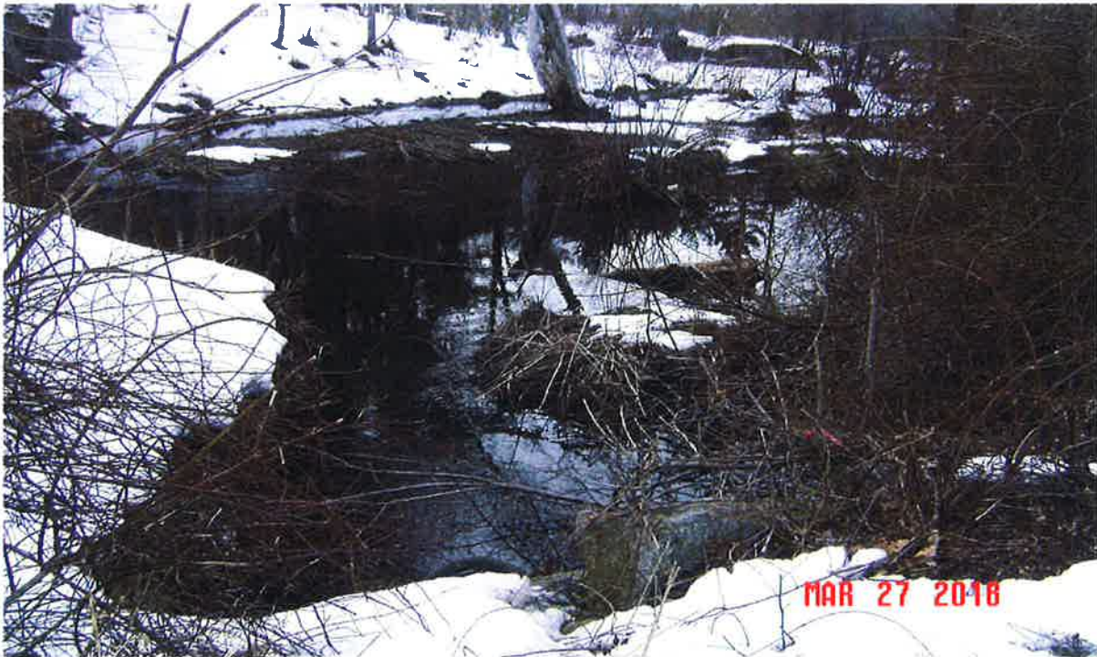
Image 22 – Looking west (upstream) from culvert D4 and Oak Street Extension. Refer to Figure 4. ©Jacobs2018
