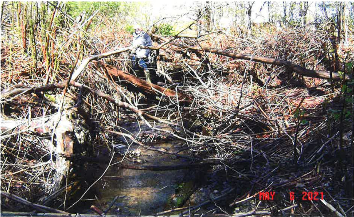
Image 18 – Looking west (upstream) at Oak St Ext & culvert D3. Note knotweed on stream banks. Jack McTigue is standing at the culvert. Refer to Figure 3. ©Jacobs2021
