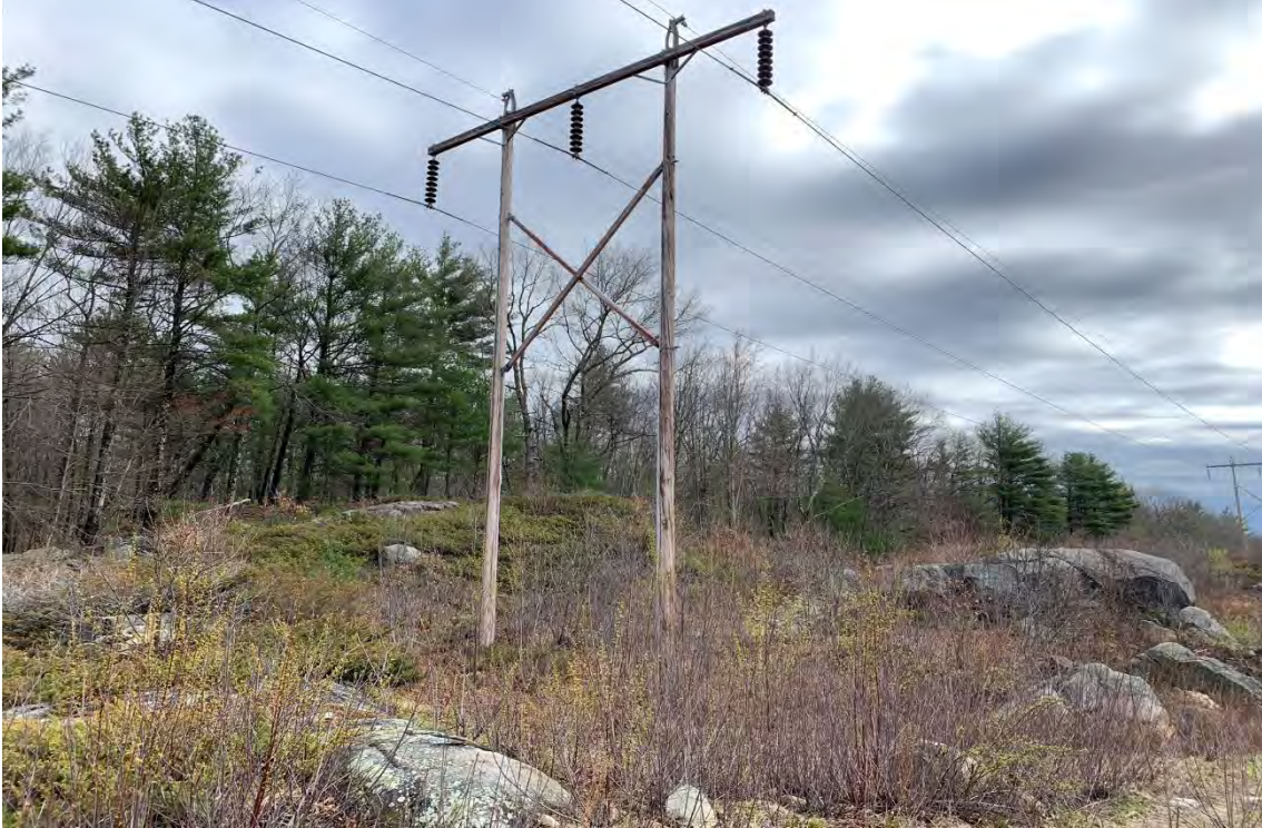
Photo 1. View northeast at existing Structure 166 proposed for replacement. Photo depicts the approximate location of temporary impacts associated with the structure work pad within the 150 foot shoreland buffer of an unnamed perennial stream that intersects the Project ROW just west of the structure.
