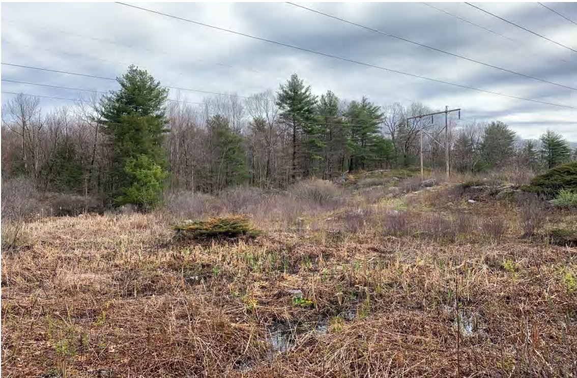
Photo 2. View northeast at Wetland EW-23. The unnamed perennial stream is not well defined as it flows through this wetland and across the Project ROW. Structure 166 proposed for replacement is depicted in the photo background.
