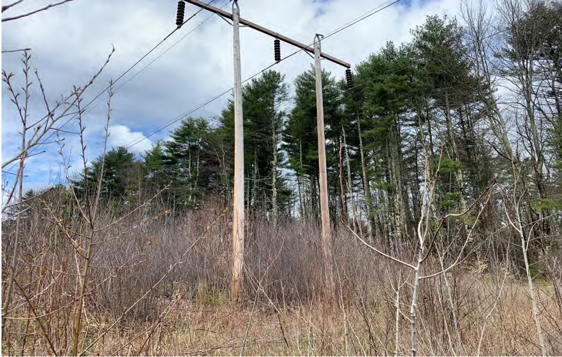
Photo 3. View northwest at existing Structure 201 proposed for replacement. Photo depicts the approximate location of temporary impacts within the 100' prime wetland buffer of Wetland EW-2 associated with the structure work pad.
