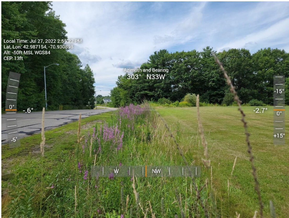
Photo: 9 – Roadside ditch diverting sheet flow to the detention-pond. Invasive species present.
