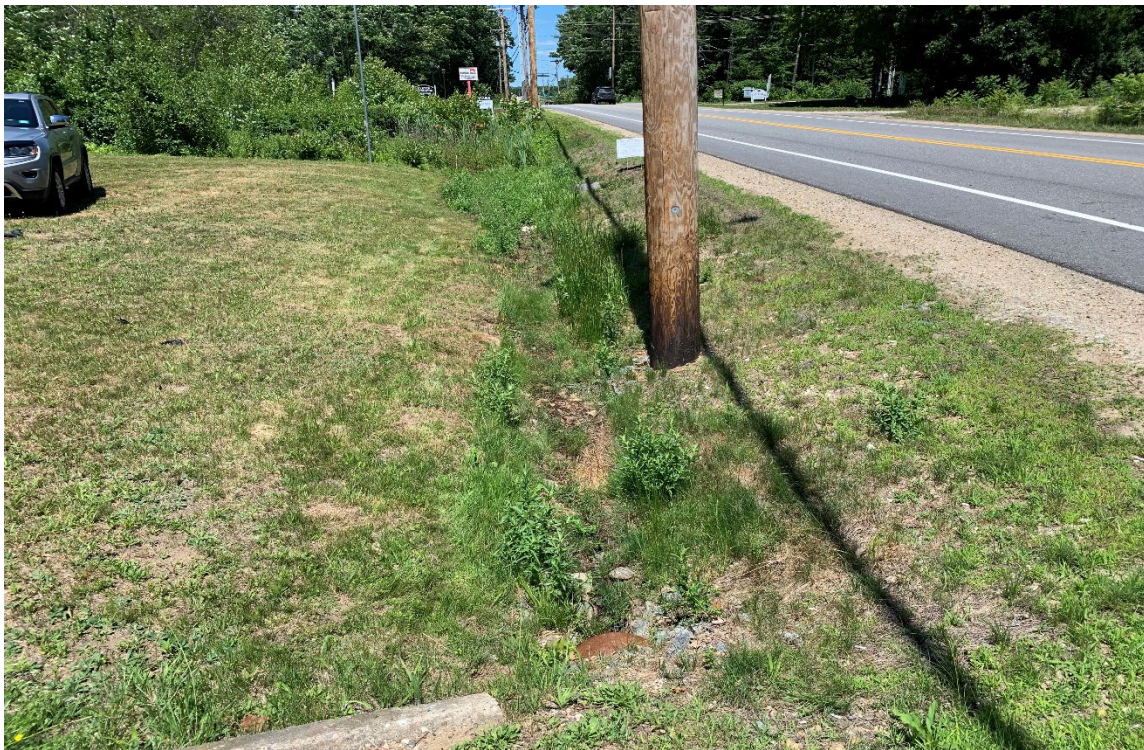
Photo 8: View north at the PEM1Cx swale portion of Wetland W-3 to the north of the existing car dealership driveway. Associated 10" CMP pipe is depicted in the photo foreground.
