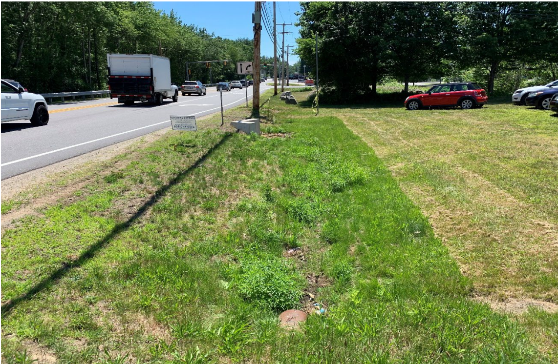
Photo 6: View south at the PEM1Cx swale portion of Wetland W-3 to the south of the existing car dealership driveway. Associated 10" CMP pipe is depicted in the photo foreground; associated 12" PVC pipe and concrete headwall is depicted in the photo background.
