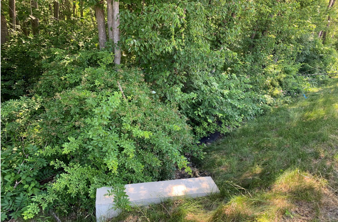
Photo 1: View southeast at existing 12" PVC drainage pipe and culvert headwall located at the toe of the existing road slope adjacent to Wetland W-1.
