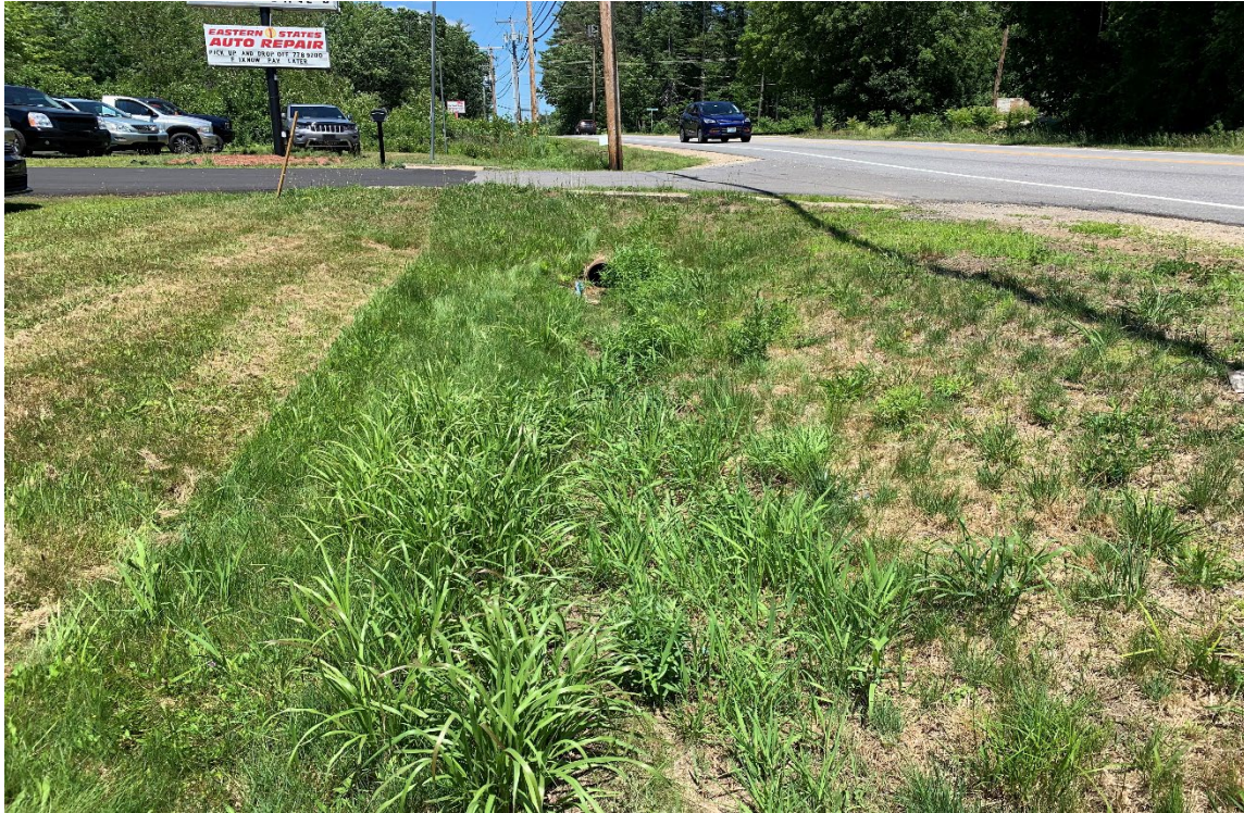
Photo 7: View north at the PEM1Cx swale portion of Wetland W-3 to the south of the existing car dealership driveway. Associated 10" CMP pipe is depicted in the photo background.
