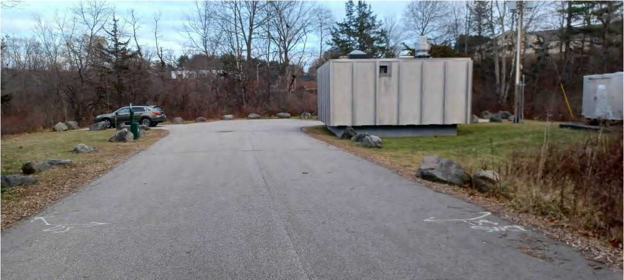
Photo 4: Taken facing easterly showing the existing pump station. Note dig safe markings on roadway showing the existing culvert location and the businesses on Route 108 in the back ground.
