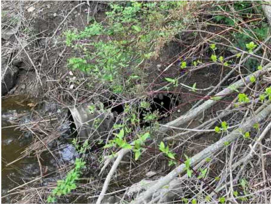
Photograph 8 – View of Culvert Running Under Webster Avenue, NW of the Webster Avenue Pump Station
