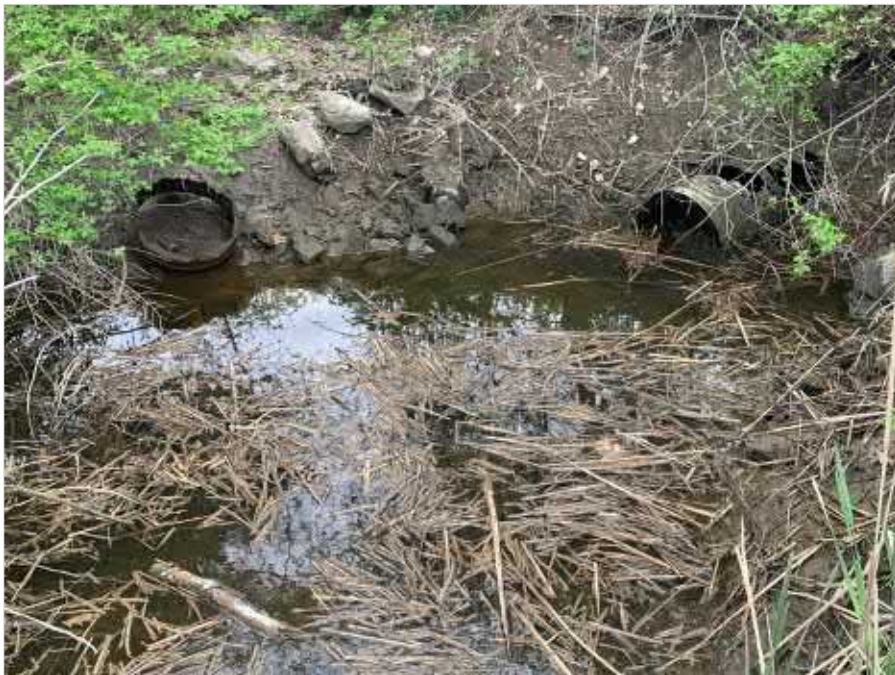
Photograph 9 – View of Culvert Running Under Webster Avenue, NW of the Webster Avenue Pump Station
