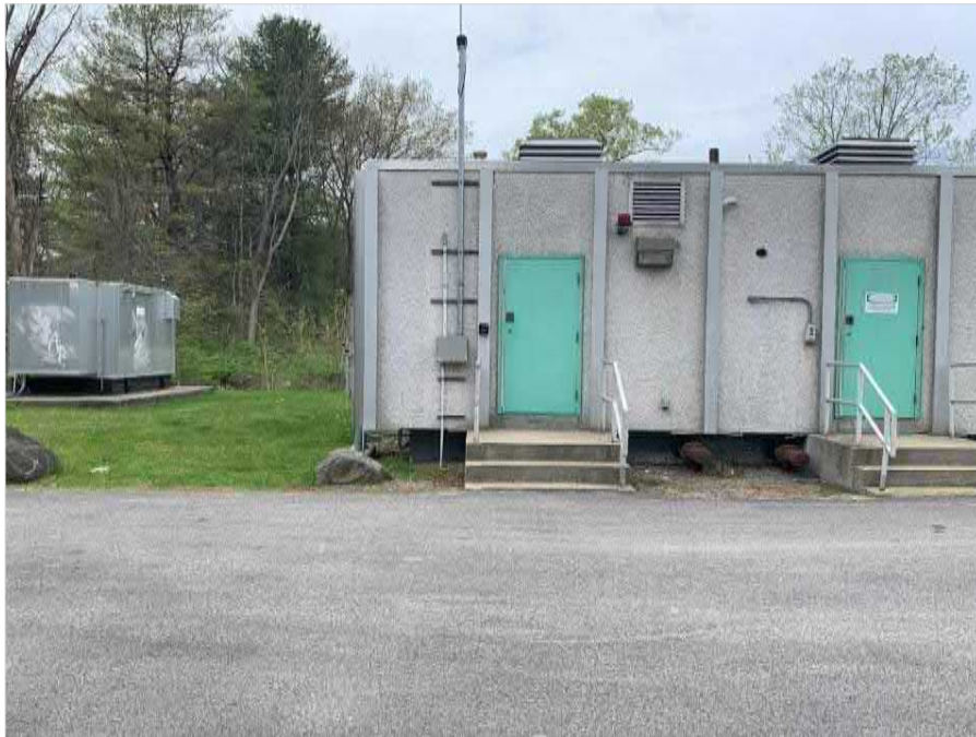
Photograph 1 – View of Existing Webster Avenue Pump Station and Standby Generator
