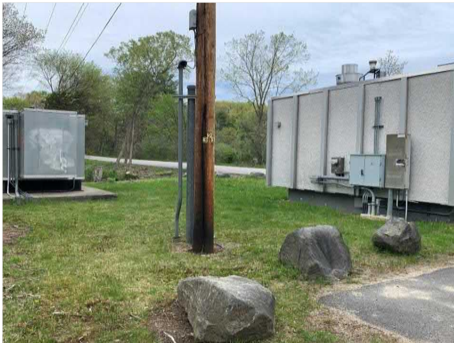
Photograph 2 – View of Webster Avenue Pump Station
