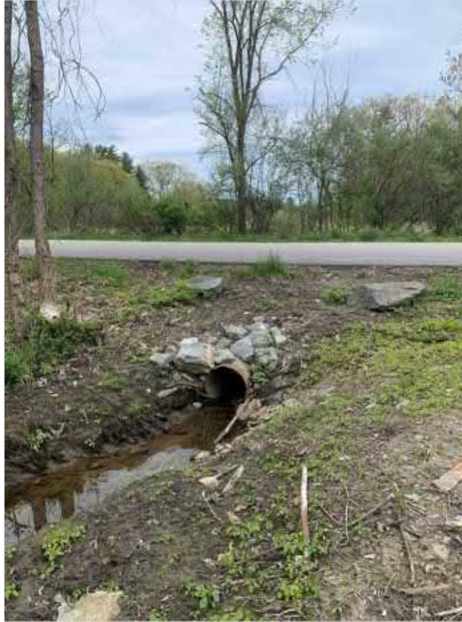
Photograph 7 – View of Culvert Running Under Webster Avenue, NW of the Webster Avenue Pump Station
