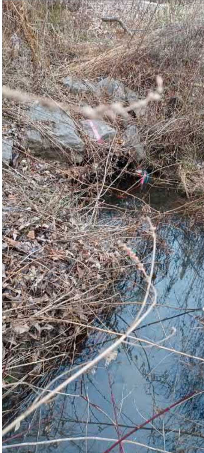
Photo 2: Showing upstream (northerly) end of culvert under Webster Avenue during a high tide.
