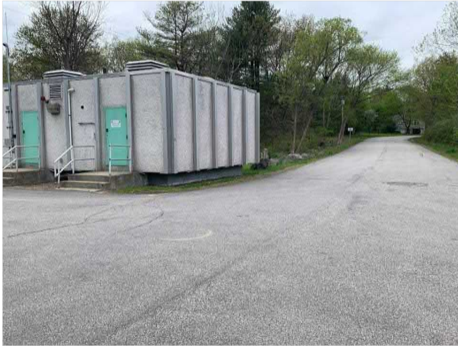
Photograph 3 – View of Webster Avenue Pump Station
