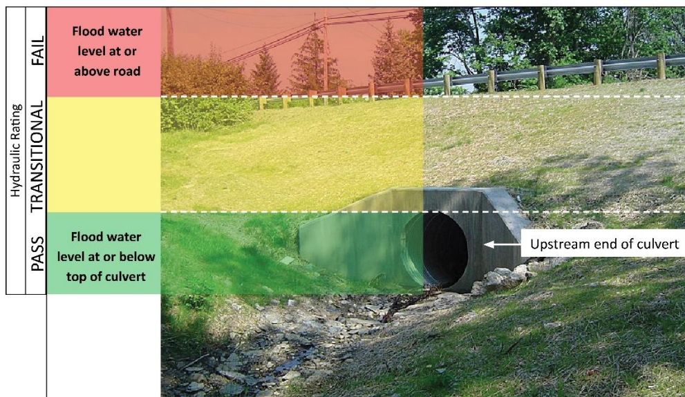
FIGURE 5: Example of how the hydraulic rating is applied to a culvert evaluation.
