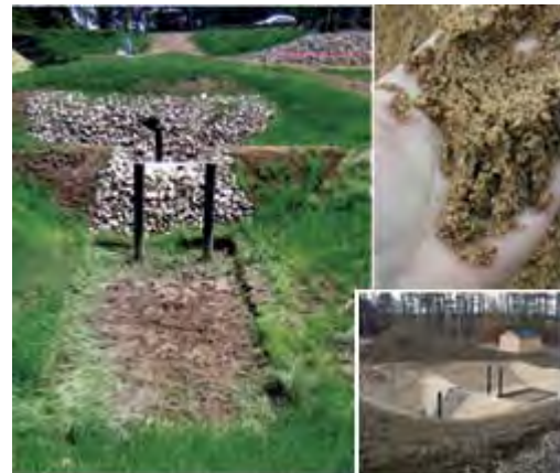
Figure 5. Sand Filter (Credit: UNHSC)
