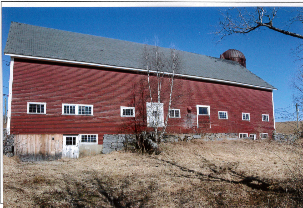
Photo # 10 Description: Milk Room Addition Removal (After) Photo 10 Milk Room Former Site:
