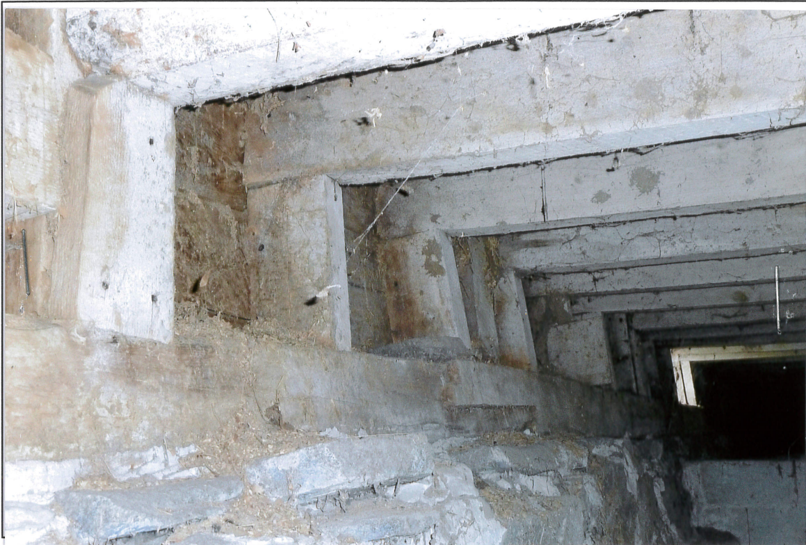
Photo # 15 Failing North Wall Sill (Before)
