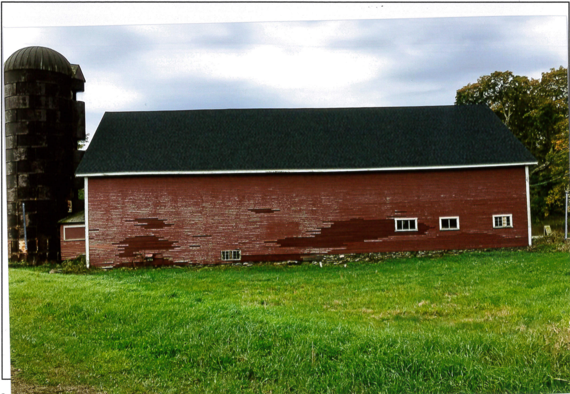
Photo # 2 Description: Area North of Barn Drainage Regrading (After) Reference Photo 2, North Drainage regrading:
