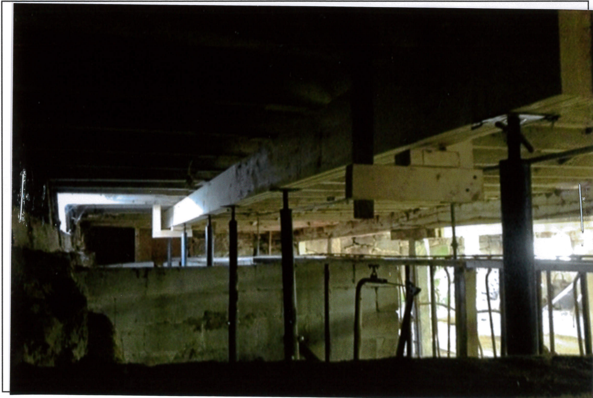
Photo # 16 Description: Failing North Sill – Temporary Stabilized (After)
