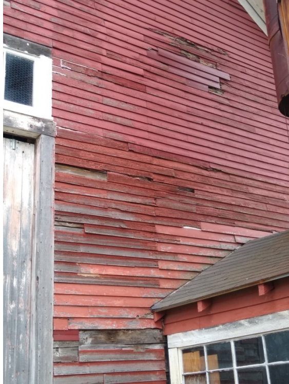
East side, northerly section with damaged, missing and replaced clapboards above connector with silo
