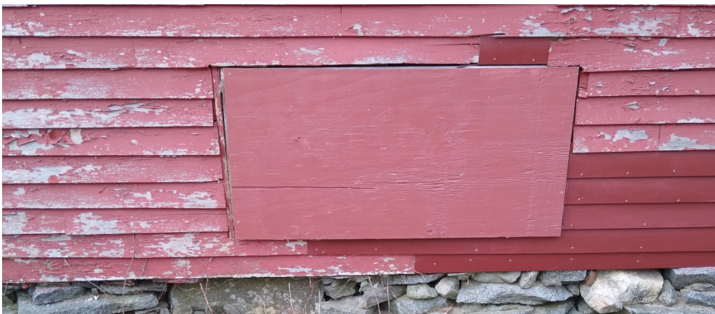
North side, middle section of clapboards showing replaced clapboards and plywood covering opening
