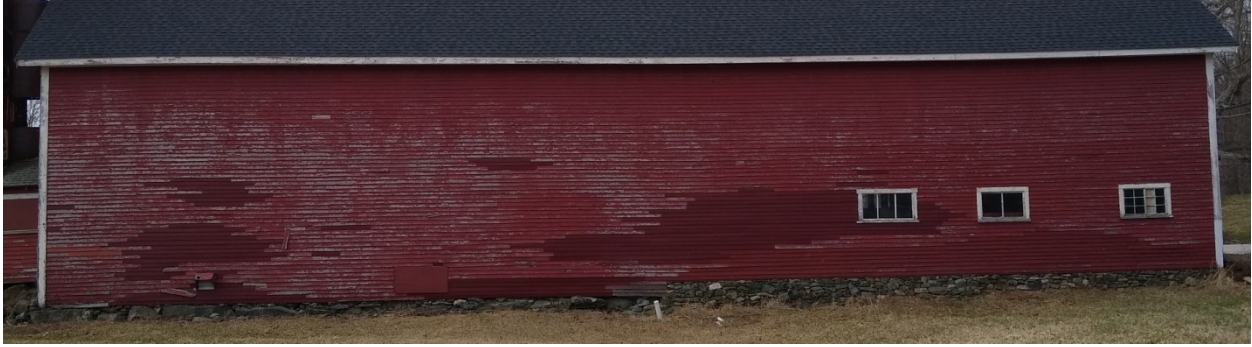
North side of barn showing a minimum of two areas of clapboard replacement as evidenced by the two newer barn red colors, "toothed-in" to the worn and lighter colored original clapboards
