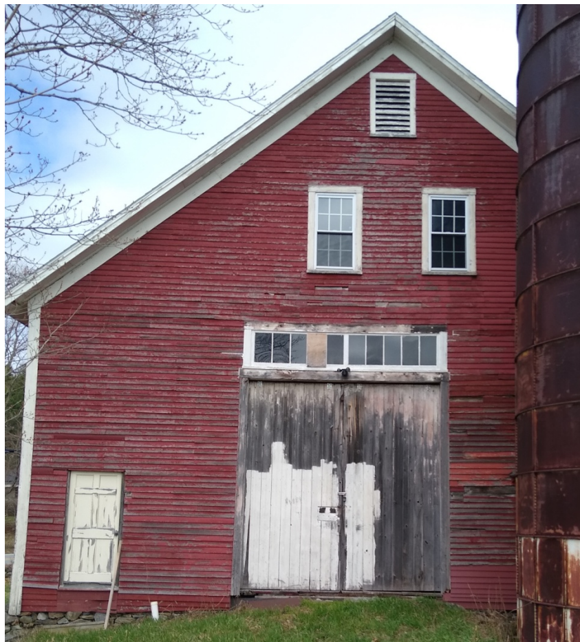
East side with damaged and missing clapboards
