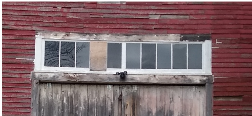
East side with damaged window and door trim
