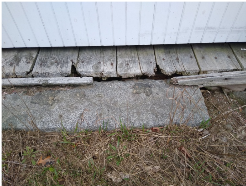
West façade, under floor at large barn doors threshold
