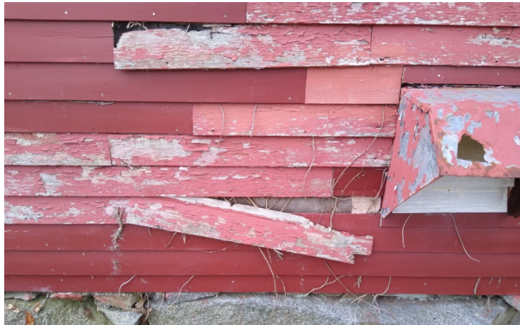
North side easterly section with clapboard repairs and damage
