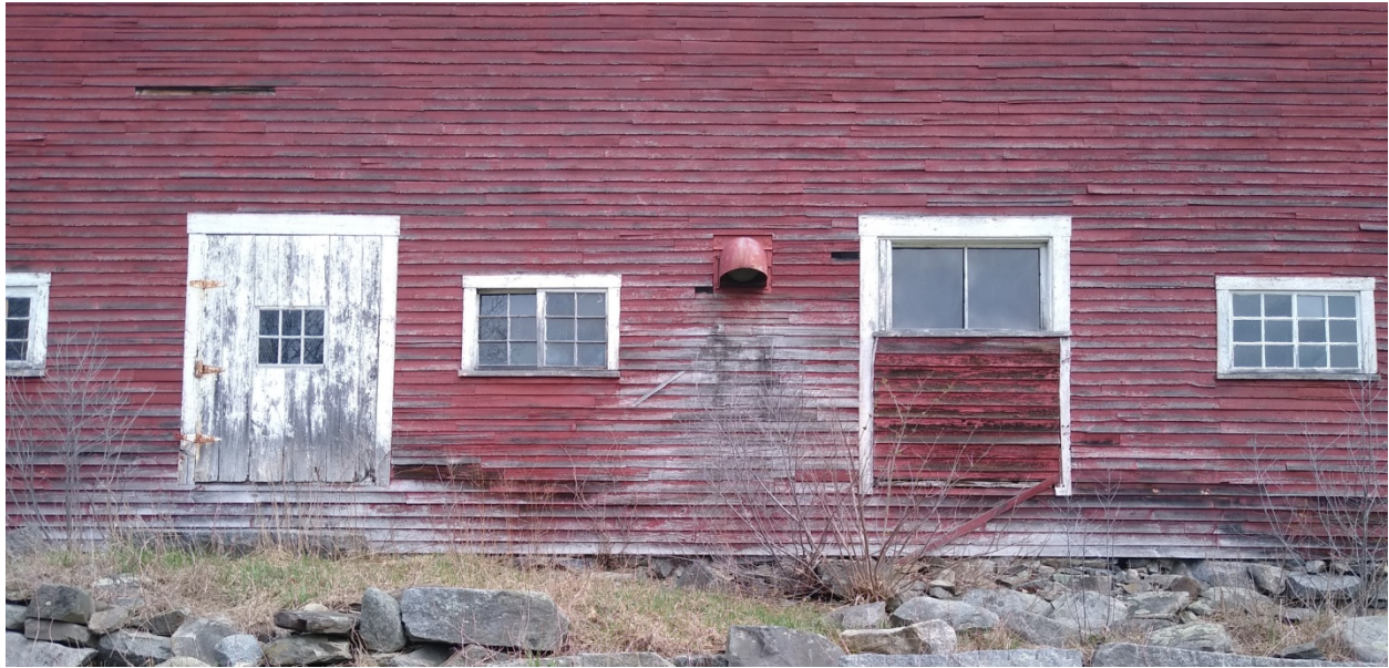
South side, middle section showing damaged and missing clapboards
