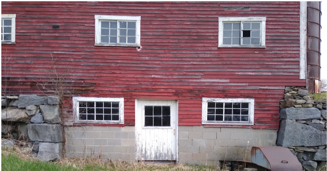
South side, easterly section showing damaged and missing clapboards with “toothed-in” clapboards in newer red paint
