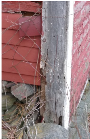
East/north corner board with deteriorated corner boards
