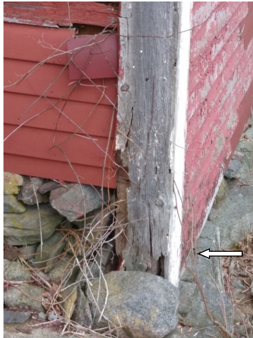
East and north corner, with the north wall (white arrow) Extending down past the height of the top of the stone foundation of the east wall (east, south and west walls are all at the same elevation)
