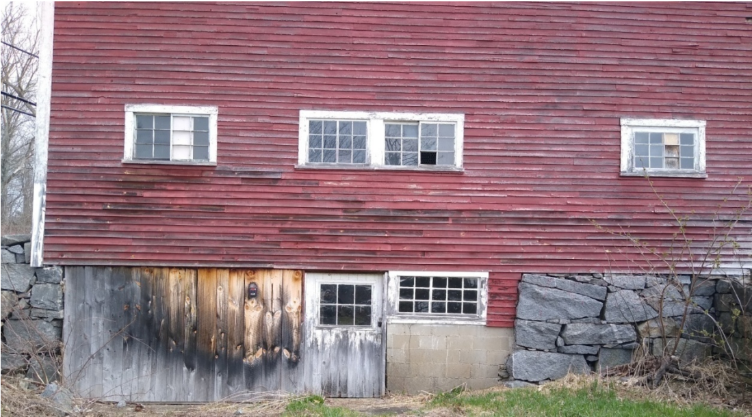
South side, westerly section with damaged clapboards, mainly above and below windows
