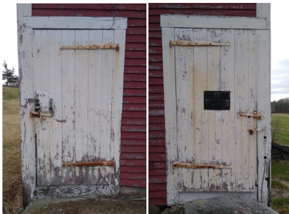
West façade passage doors on both sides of the large barn doors
