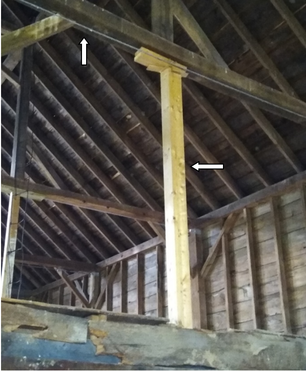
Looking northwesterly, steel cable (upward arrow) added support beam (left hand arrow)
