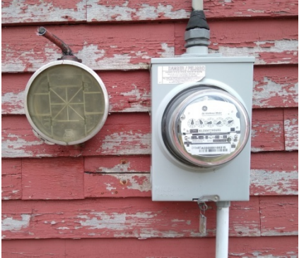
West Façade, with old meter box on left and new meter box on right
