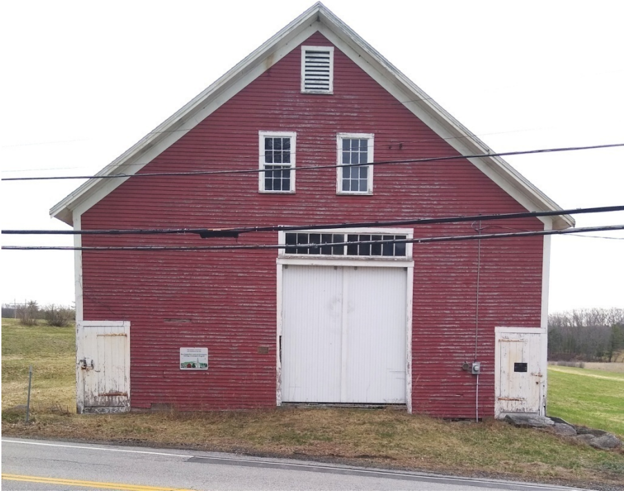
West façade with minor clapboard damage/loss
