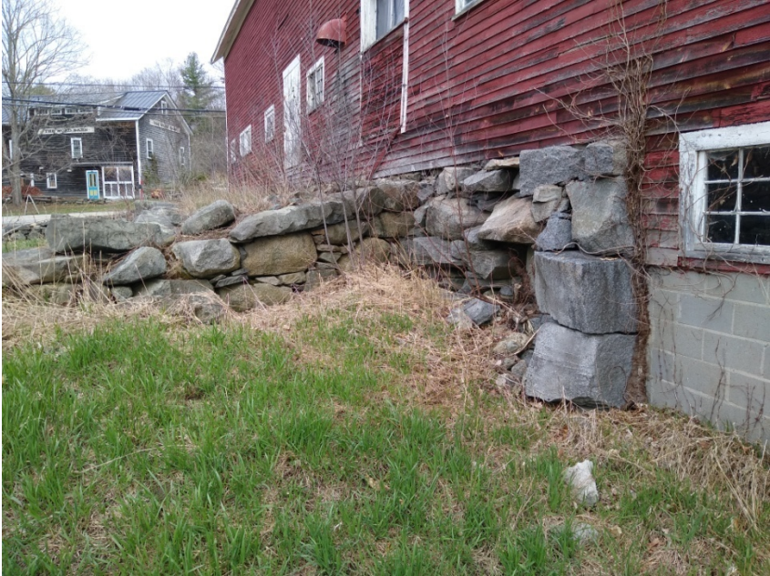
Eastern side of south ramp with brush growing along the foundation
