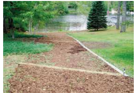
Waterbars along the path slow flow and divert runoff into the vegetated area.
