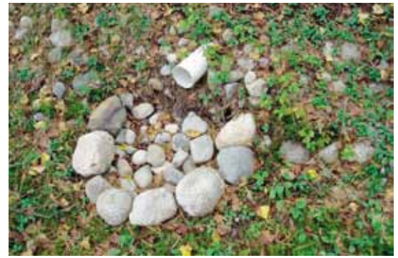
A plunge pool is an area where water is collected and allowed to infiltrate.
