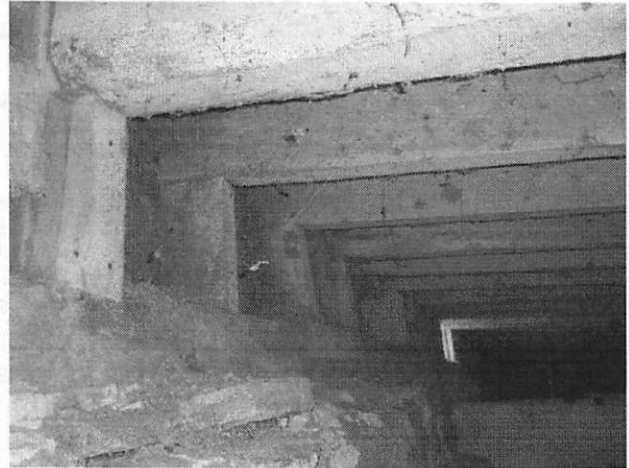
Bowing North Sill
