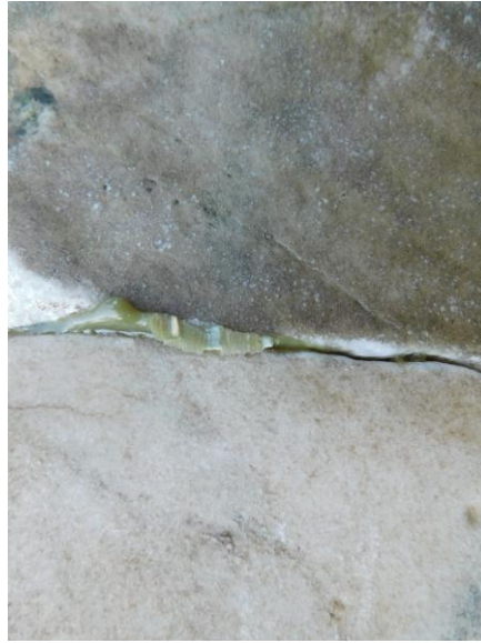
10. EWSC. A108. DT. Detail of excess epoxy.
