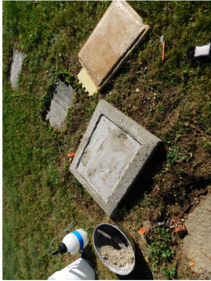
10. EWSC. A109. DT. Overview of granite and marble ready for setting in mortar.
