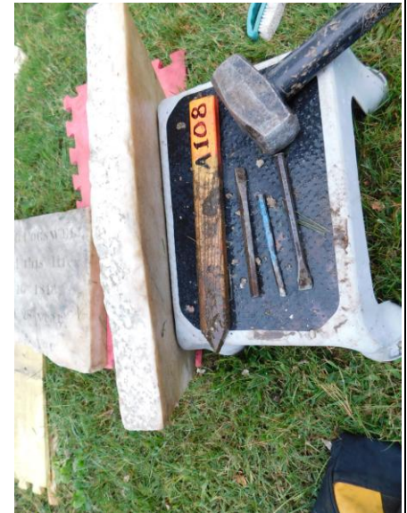
8. EWSC. A108. DT. Removal of failed bonding cement with hammer and chisle and Dremel.
