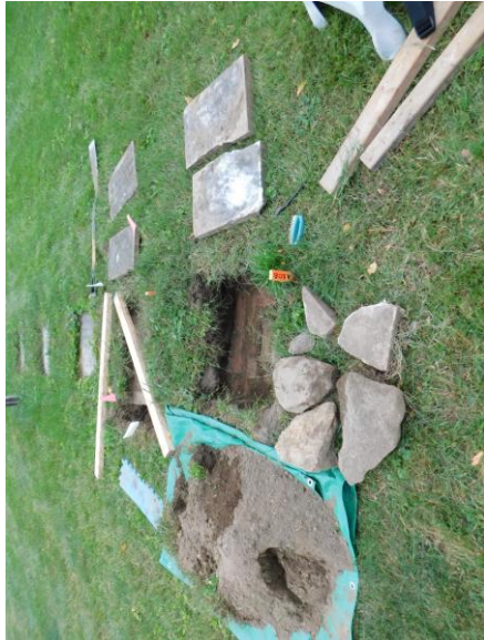
3. EWSC. A108. DT. Overview of area after removal and removal of foundation materials.
