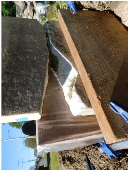
7. EWSC A22. DT View of loss before fill.
