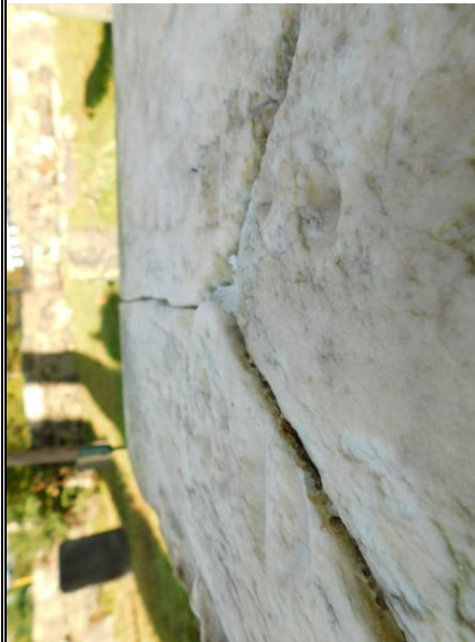
7. EWSC. A29. DT. Detail of misaligned previous repairs with adhesive mortars.
