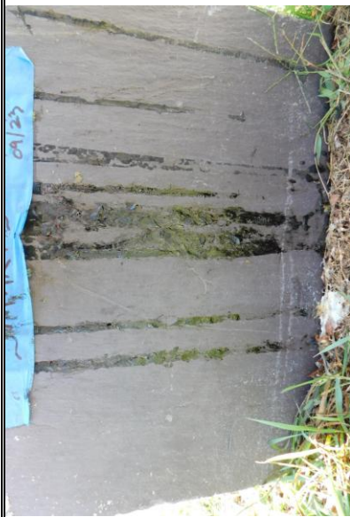
7. EWSC. F80. DT. View of first stripping test. Thick accumulations were removed with popsicle sticks.
