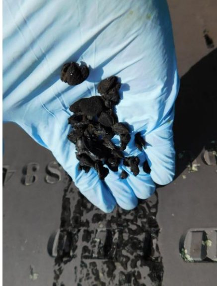
16. EWSC. F80. DT. Holding tar scappings from front of slate.
