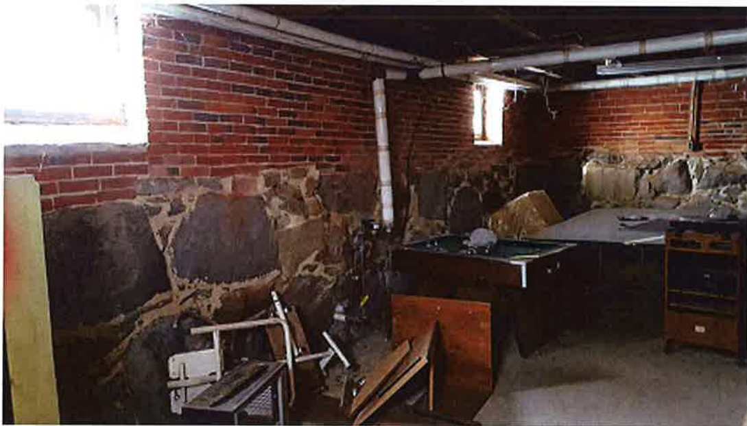
IMAGE 6 - 8 GILMAN LANE BASEMENT. NOTE THE BRICK FOUNDATION, SHOWING THAT THE HOUSE WAS RAISED UP AT SOME POINT IN TIME.
