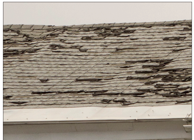
This 3-tab asphalt shingle roof has exceeded its useful life. Given the unevenness of the surface, it would be prudent to have the underlying framing and sheathing reviewed by an architect or engineer prior to re-roofing.
