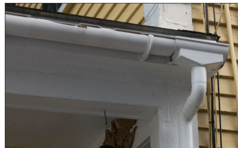
The water from this half-round gutters is collected in a scupper box and directed to a round downspout. All are painted white to match the wood trim.
