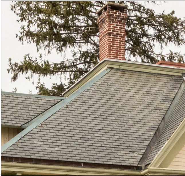
Slate roofing is often found on Exeter's older buildings. Also note the copper flashing along the roof hip.
