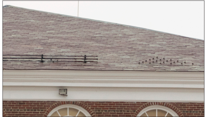
This slate roof has two types of snow guards along the roof eave, spaced brackets supporting metal rods above, the left and individual guards to the right.
