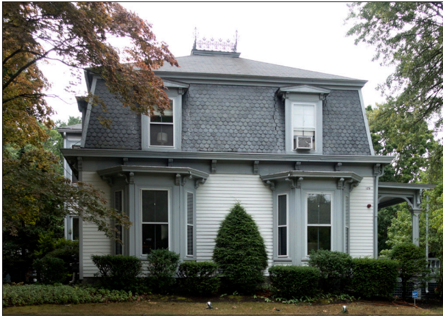
Mansard roofs are common features of Second Empire buildings. This slate mansard roof features decorative cresting at the uppermost roof level.
