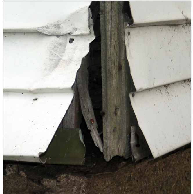
Aluminum and vinyl siding were sometimes installed to conceal an underlying problem. In some cases, removal might be necessary to repair a deteriorated condition.
