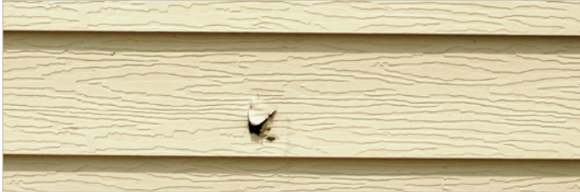
Replacement of this aluminum siding is the best way to repair this puncture. A wood-grained texture is inappropriate.
