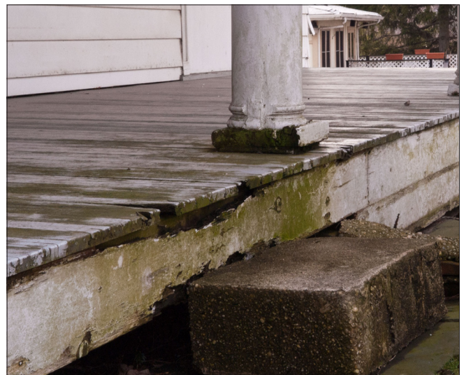
Porches, steps and other areas where the woodwork is laid horizontally or located close to the ground are often the first to deteriorate. Ongoing exposure to moisture can lead to rot of the column bases, porch deck and apron.
