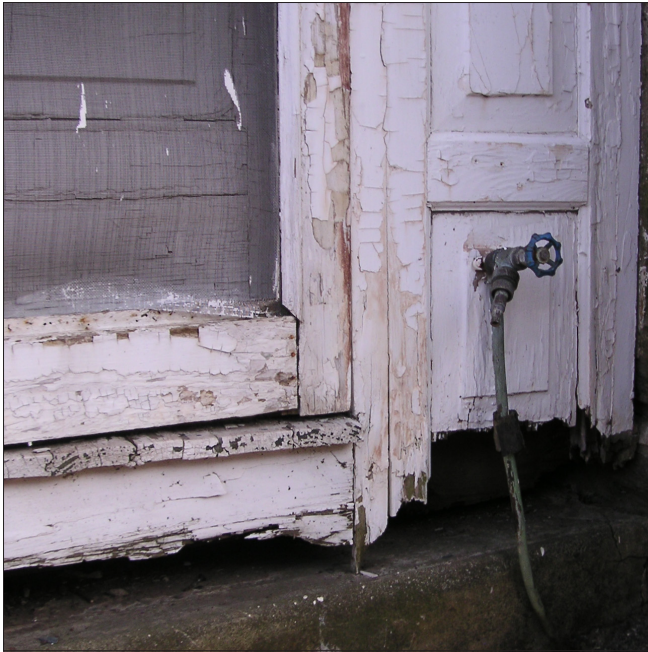
Leaking plumbing, including exterior hose bibs, can regularly expose woodwork to moisture, eventually resulting in rot. Wet wood can also be a desirable home for pests such as termites.
