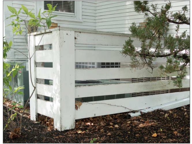
Ground mounted equipment can often be screened with fencing or shrubs to minimize its visibility.
