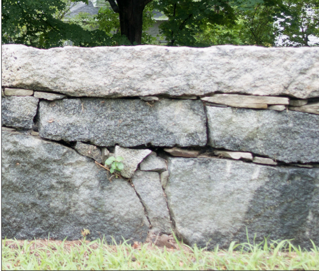
Granite, which is readily available in Exeter, is a very durable material that is ideal for the construction of landscape walls. This dry-laid granite wall includes larger stones held in place by smaller ones, all topped by a relatively flat capstone.
