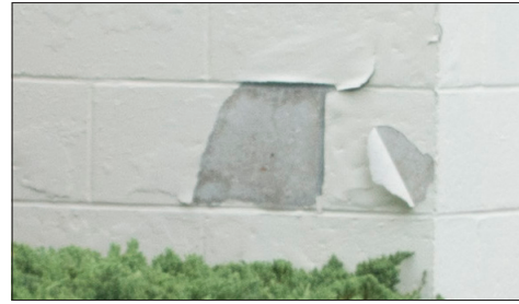
Badly peeling paint can be an indication of poor preparation or moisture issues.
