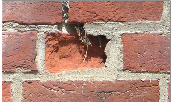
The surface of the center brick has spalled. The repointing mortar is harder than the brick and likely includes too much Portland cement. The mortar should be completely replaced with softer mortar.
