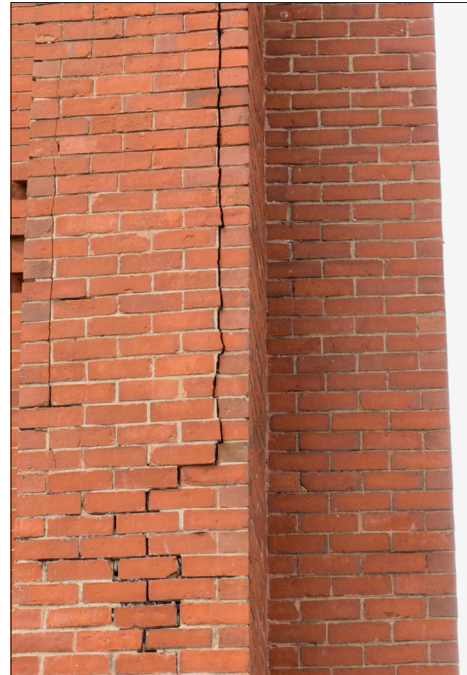
Long cracks at masonry, particularly cracks that split individual cracks or stones, can be an indication of a significant structural problem. In cases of more significant or re-occurrent cracking, consultation with an architect or structural engineer may be prudent prior to repointing.
