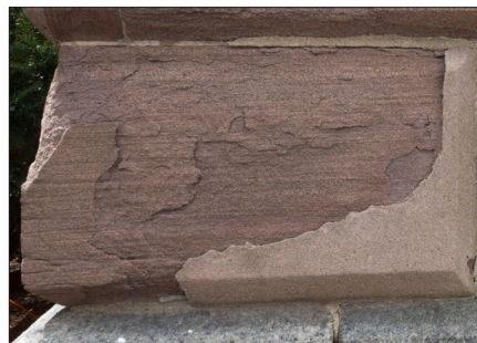
Brownstone is very soft and susceptible to moisture damage. The surface of the brownstone has delaminated, the corner has spalled and a cementitious patch on the lower right corner is failing.
