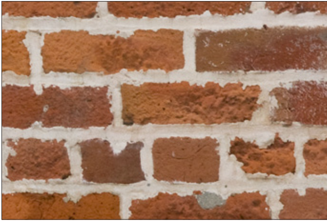
A saw was used to cut-out the joints during repointing, extending the vertical joints and damaging the bricks. In addition, both the vertical and horizontal joints have been widened.
