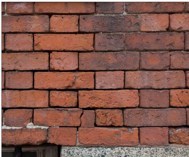
The mortar has weathered from most of the brick joints, reducing the structural capacity of the wall. The surface of some bricks has spalled, and a settlement crack has developed near the corner of the window.
