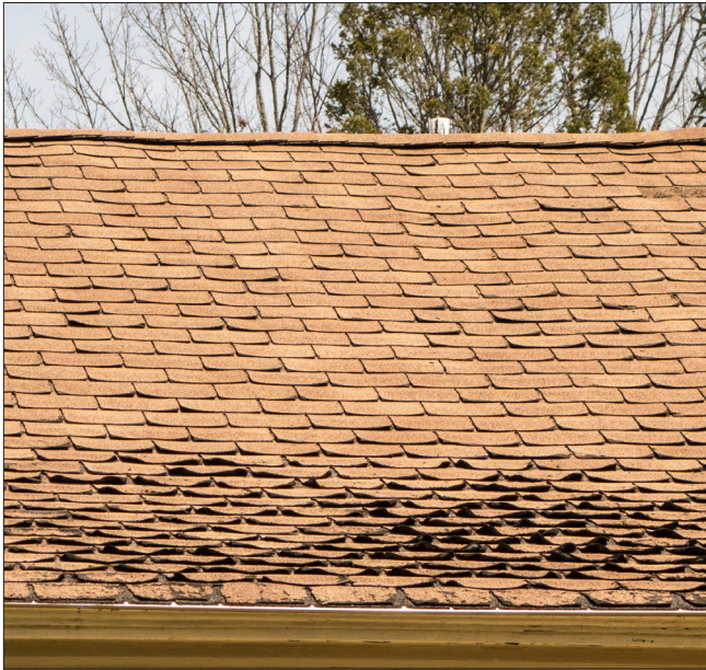
The replacement of deteriorated roofing is potentially dangerous work that often requires the access of workers and materials by ladders. Consideration should be given to hiring a professional for any work that is unfamiliar or potentially unsafe.
