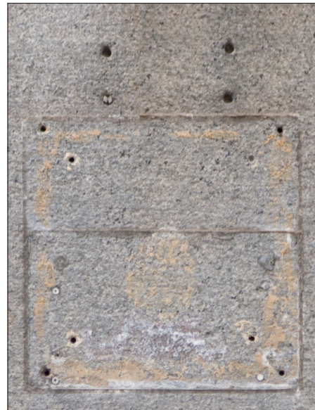
Numerous holes have been drilled into the face of this granite pier and several abandoned fasteners still remain. Fasteners should be removed, existing holes reused for future signs, abandoned holes filled and the stone surface cleaned. (Refer to Guidelines for Masonry & Stucco.)
