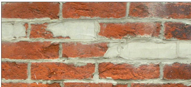
The rough texture and uneven surface suggest an aggressive cleaning method was used. Stucco patches replace bricks and efflorescence, a white powdery substance, can be seen on the surface.
