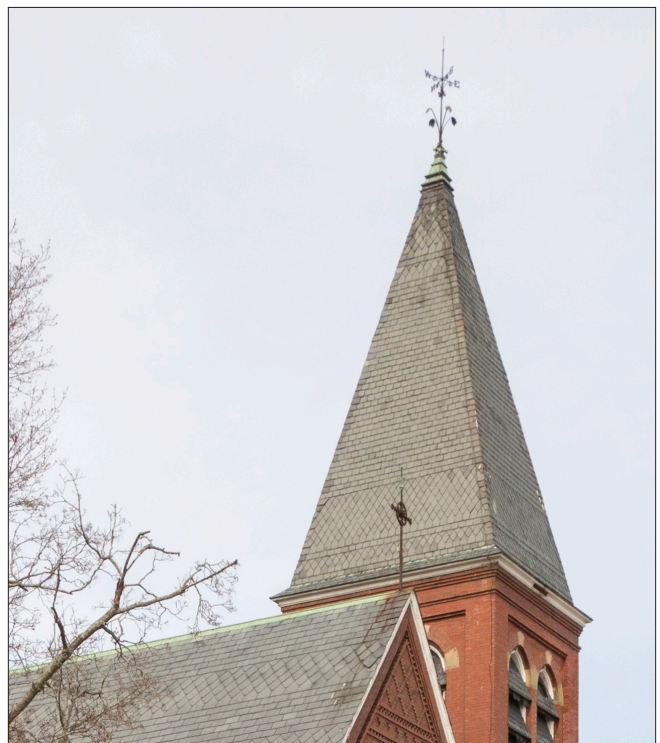
Roof forms can provide a dramatic building silhouette against the sky. Both the pyramidal hipped roof of the tower and the front gable roof have bands of patterned slate, typical of the Victorian period.
