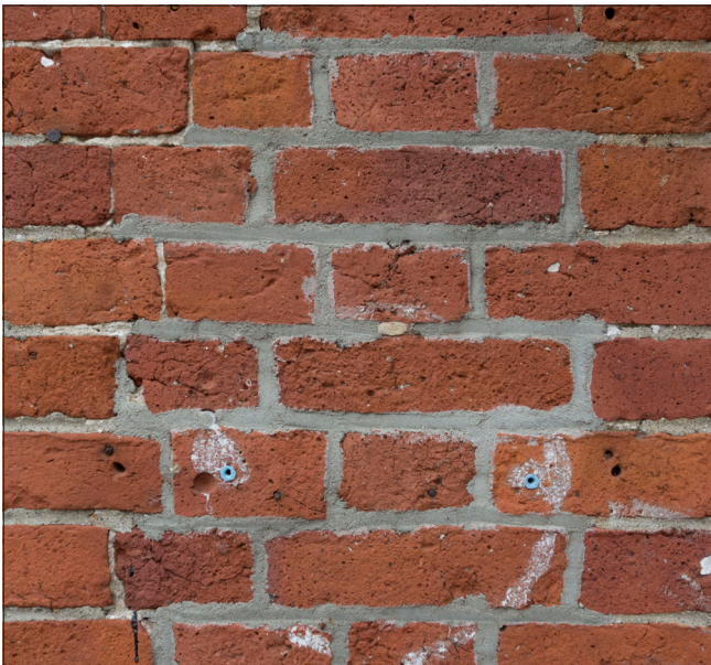
The central bricks have been repointed with what appears to be a Portland cement mortar that is harder than the hand made brick. In addition, the mortar color and tooling is a poor match for the original mortar.
