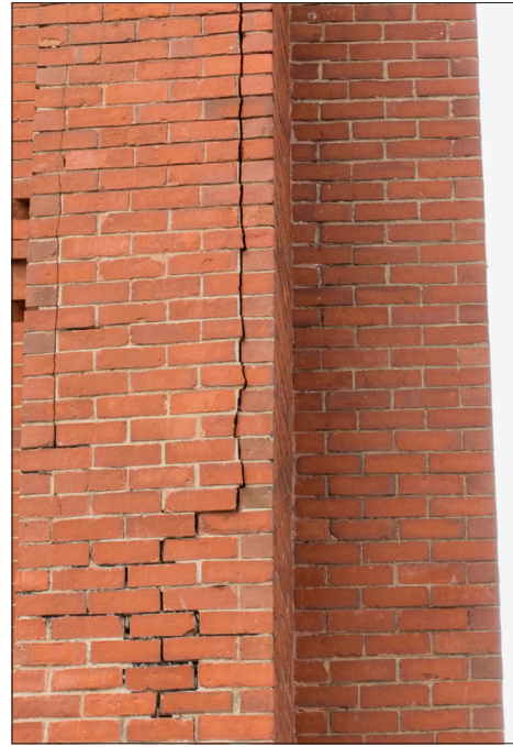
Long cracks at masonry, particularly cracks that split individual bricks or stones, can be an indication of a significant structural problem. In cases of more significant or re-occurrent cracking, consultation with an architect or structural engineer may be prudent prior to repointing.
