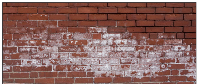
Efflorescence, or white bloom, is an indication of moisture in the wall. There is a lack of mortar at the upper right.
