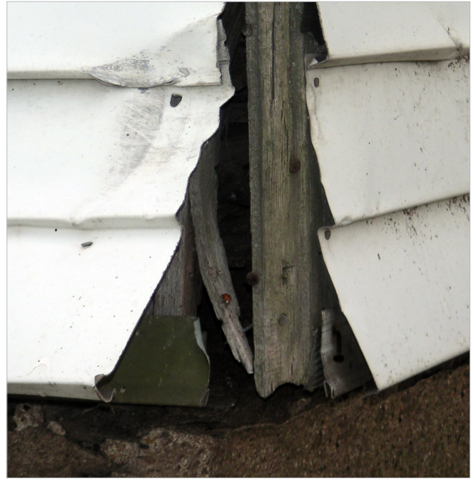
Aluminum and vinyl siding were sometimes installed to conceal an underlying problem. In some cases, removal might be necessary to repair a deteriorated condition.
