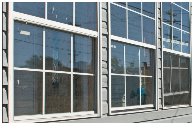
Vinyl windows with applied muntins lack the profiles and details of traditional wood windows and are not appropriate at historic buildings. They are also mounted flush to the outside wall without trim or casings.
