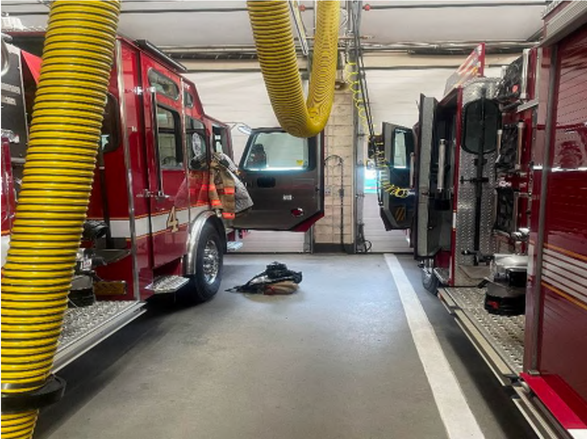
Figure 8- Limited space Between Parked Apparatus – This space limitation can delay response, plymovents strike adjacent apparatus when they disengage from responding units. A lack of traction-based flooring provides the potential for injury.
