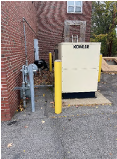
Figure 16 – Unsecured utilities and backup generator
