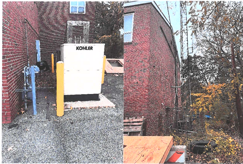
Generator and fuel source (L), and the radio antenna/transmission lines (R) are accessible to tampering.
