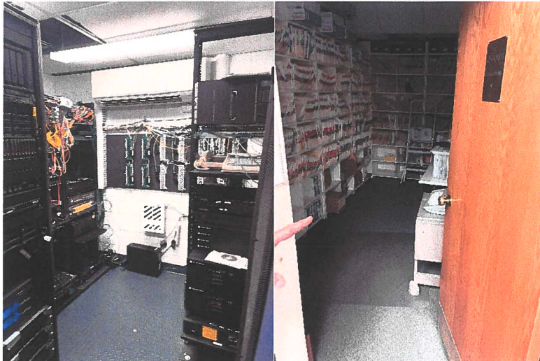
Electronic records for multiple departments in town government are retained within this server room (L). Some hard copy records for the police are retained in this secure room which is near or at capacity (R).
