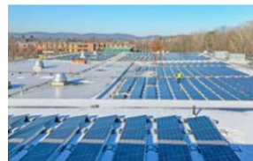
City of Keene Police Department & Public Works Building 643 kW (2018)
