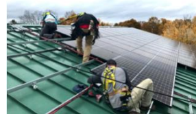
City of Nashua Transit Garage, Fire Station, Ice Arena 1.6 MW (2019-20)
