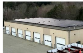
Town of Hanover Water Department, WWTF, 5 Rooftops 2 MW (2016-21)
