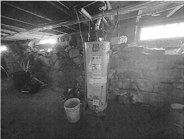
Description: Propane water heater.
