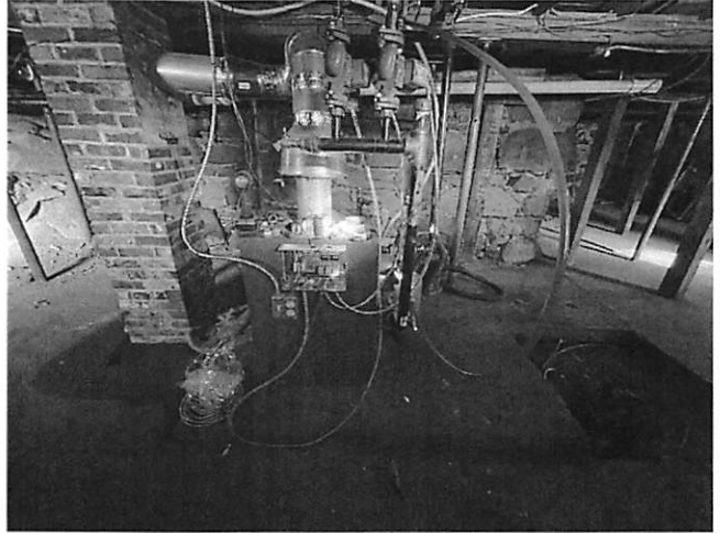
Description: HVAC system.
