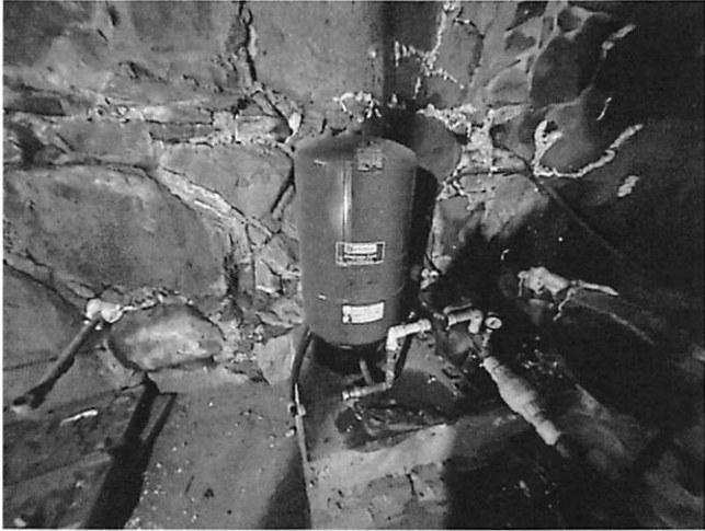
Description: Diaphragm tank.
