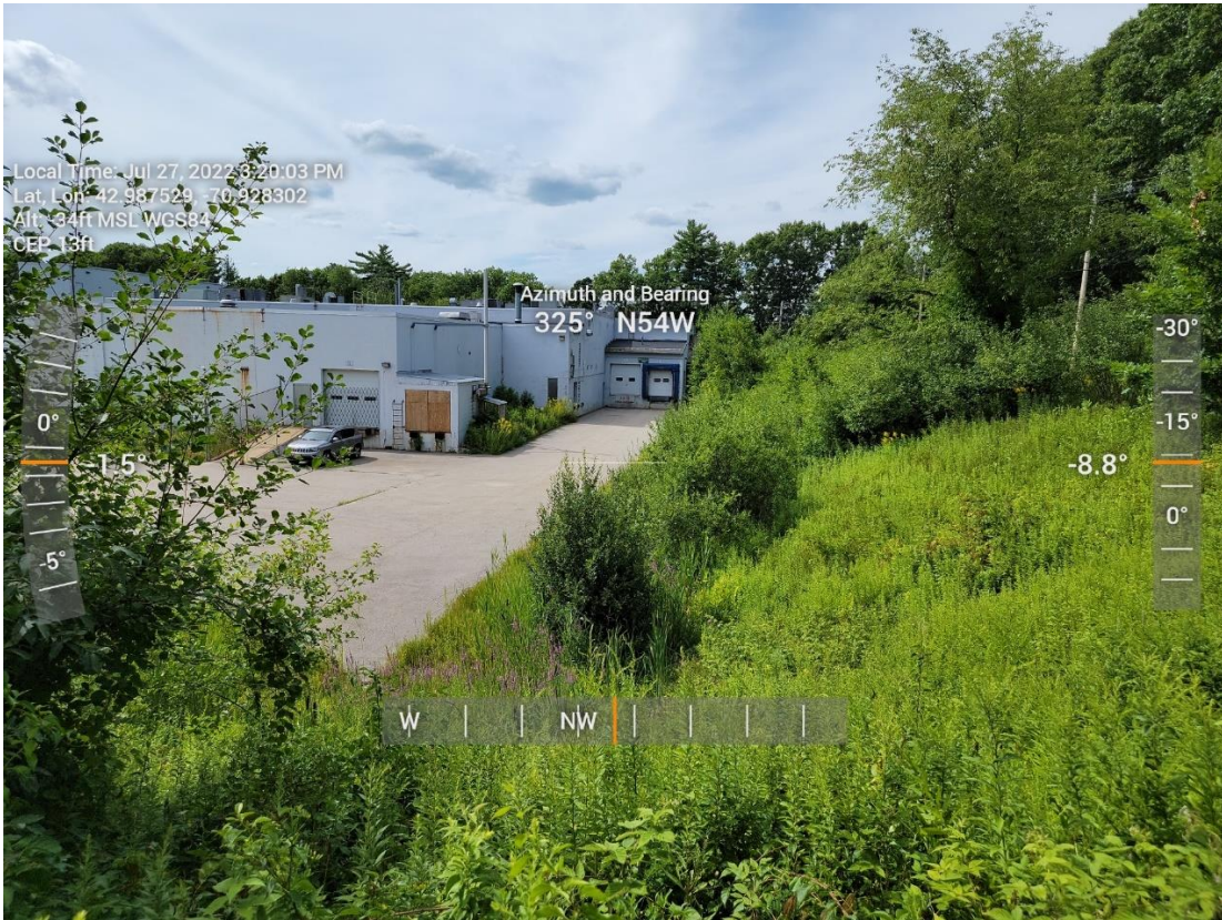
Photo: 3 – Low functioning, low value ditched area at toe of slope with invasive species.
