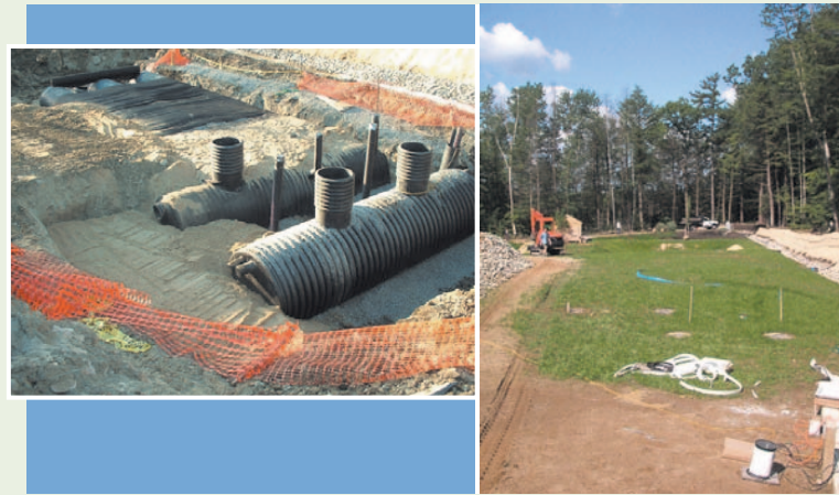
The ADS treatment system during [left] and after installation [right]. Stormwater is pretreated for sediment and floatables in the black HDPE pipes, and then flows into the adjacent storage infiltration unit, where a sandy subbase is critical to pollutant removal.
