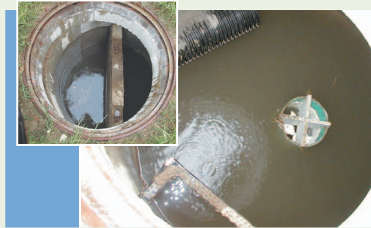
The V2B1's first chamber [right] uses a hydraulic vortex to settle out particles, and then allows clarified water to exit through a central drain into the second chamber [left], where a baffle traps oil and organic debris.
