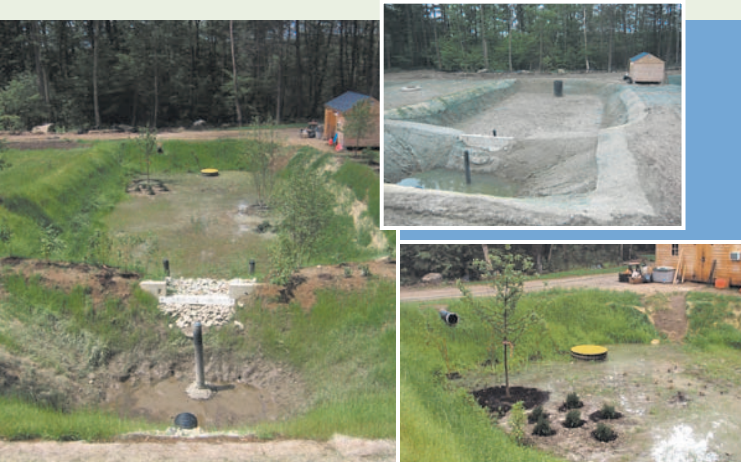
Hydroseeding and erosion control matting protect this system after installation [center]. Native species were planted along the installed system's [left] forebay and bioretention cell. Vegetation and appropriate soil media combine for effective water quality treatment [right].
