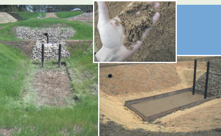
The coarse sand [center] used in this surface sand filter [left] provides physical and chemical water quality treatment. Erosion control matting protects the treatment after installation [right] until surrounding slopes are vegetated.
