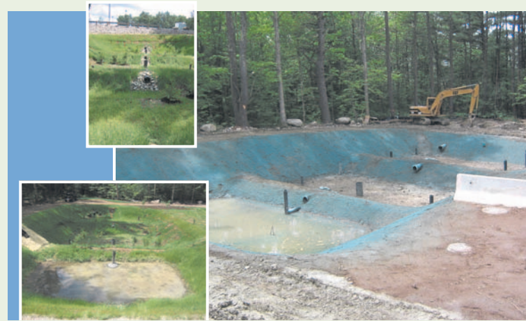
The fully vegetated gravel wetland [left top & bottom] exhibits excellent pollutant removal, provides subsurface anaerobic treatment, attenuates peak flow, and reduces flow volume. [Right] The gravel wetland's forebay and retention cells just after installation.
