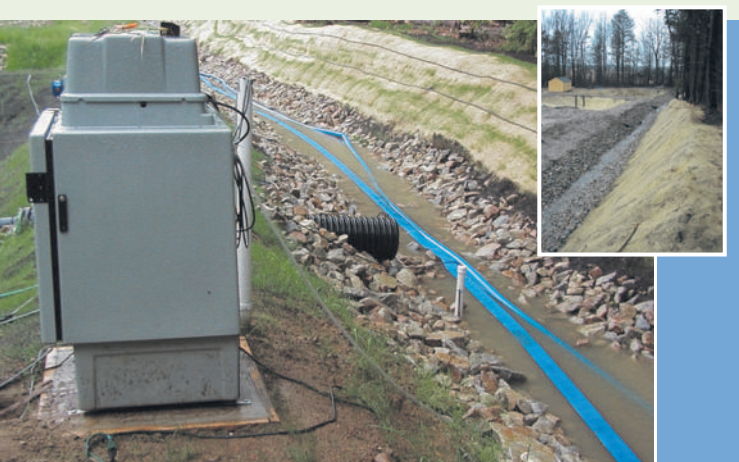
The stone swale [right] is designed to mimic a natural stream channel. Its combination of rock and fabric [left] helps trap sediment and promote vegetation. This treatment performed poorly for most evaluation criteria.
