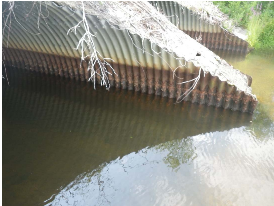
Typical culvert wall rusting at the water line
