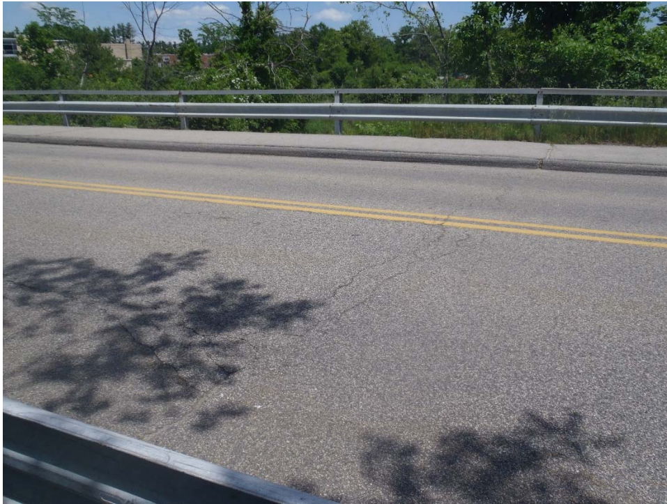
Cracking in roadway and sidewalk pavement parallel to culverts
