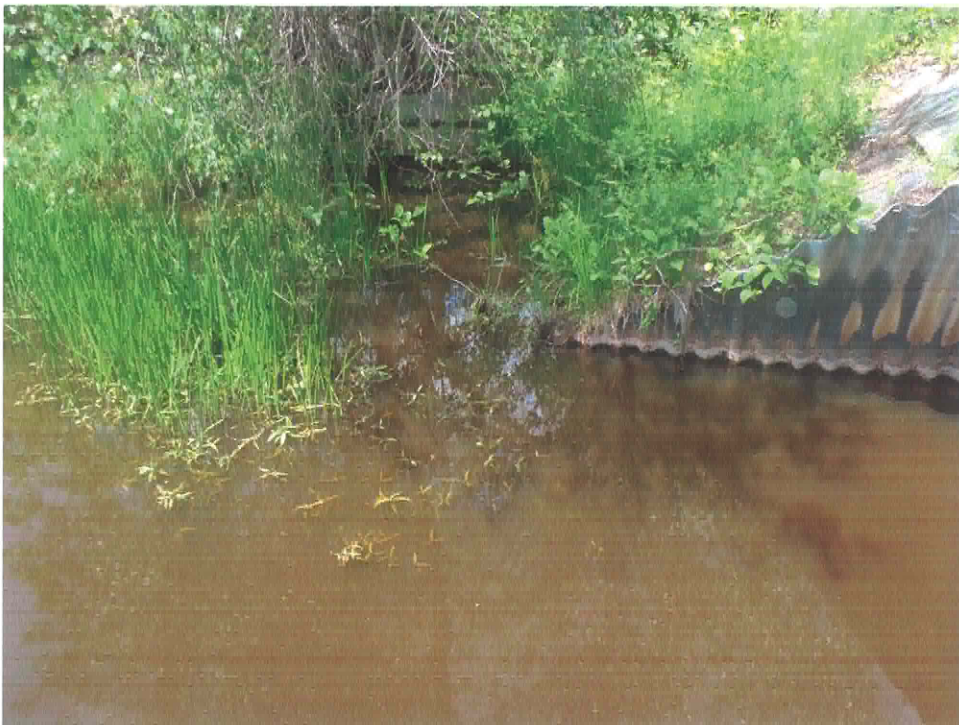
Typical culvert wall rusting at northerly culvert
