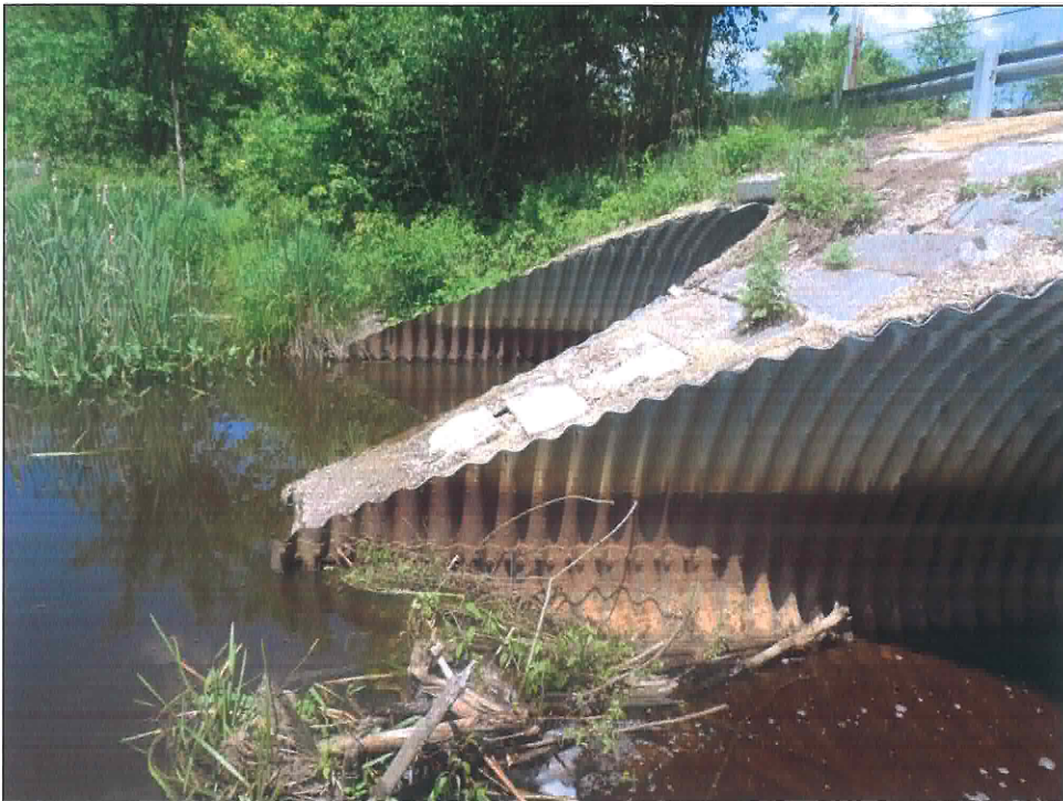
Typical culvert wall rusting with debris in the southerly culvert
