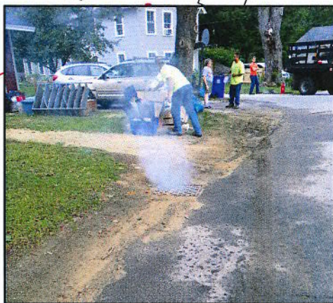
HEAVY SMOKE FROM DRAIN CONNECTION TO THE SEWER
